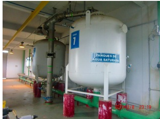
8. Saturation Tank of Irai WTP
