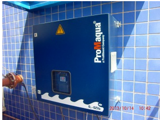
16. Pilot plant of advanced treatment in Irai WTP (ozone generator)
