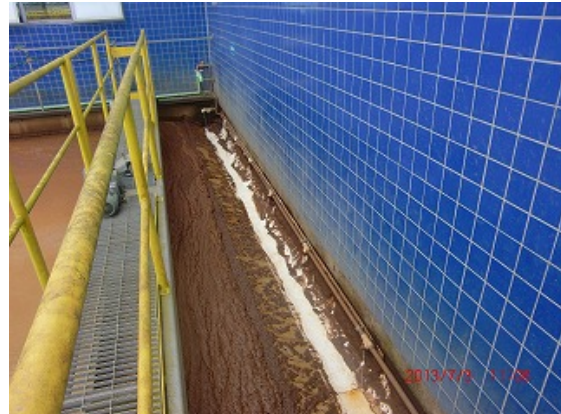
10. Floating sludge removal system of Irai WTP
