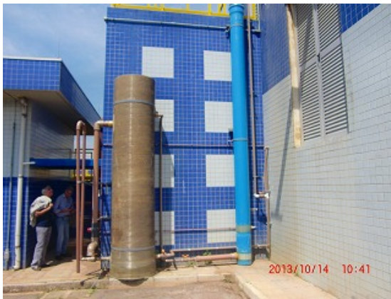
15. Pilot plant of advanced treatment in Irai WTP (right: ozone contacting tank; left: granular activated carbon filter)
