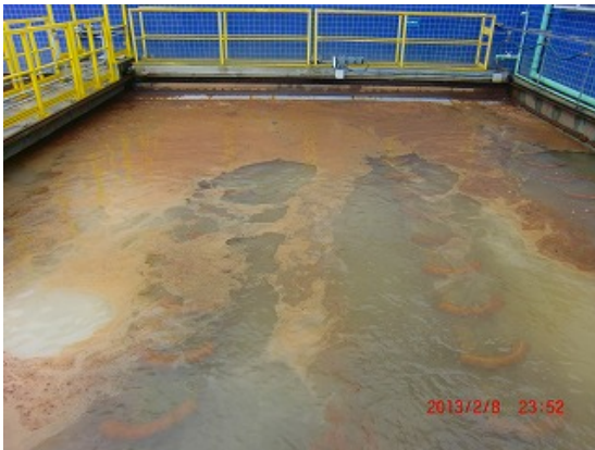
9. DAFF (Dissolved Air Flotation in Filtration) system of Irai WTP
