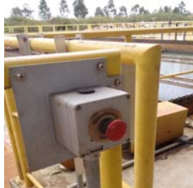
Image 67 - Scraper emergency button
