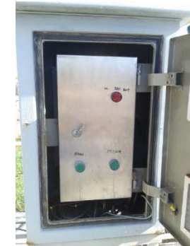
Image 56 - Bypass sluice panel
