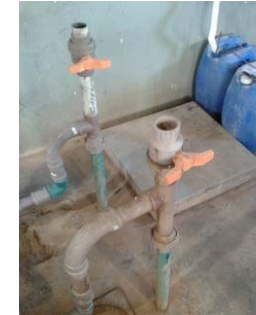
Image 94 - Hatchway of the utilities water well
