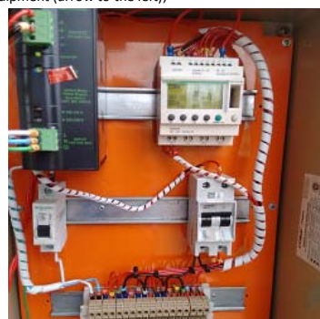
Image 69 - Inside Zelio command panel
