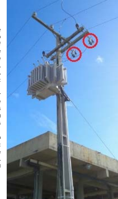
Image 103 - Pole with cutout fuse (floaters 01)
