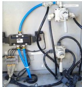
Image 55 - Command panel of pneumatic sluices
