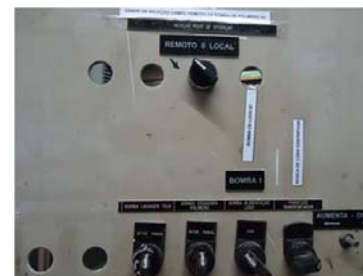
Image 88 - Detail of the command panel
