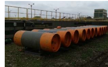
Image 10 - Chlorine Application System
