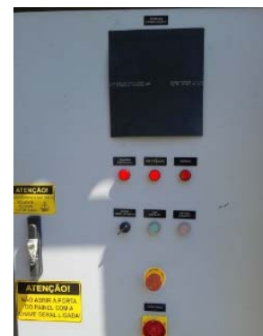
Image 21 – Command panel of automated grates
