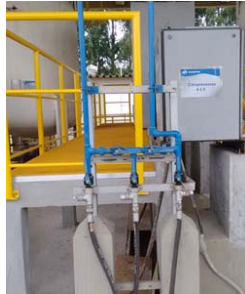
Image 72 - Valves of the compressed air pipeline
