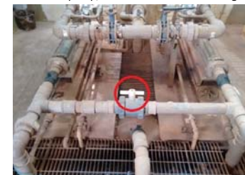
Image 83 - Sludge pipeline valve
