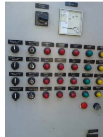
Image 19 – RSPS's sluices command panel
