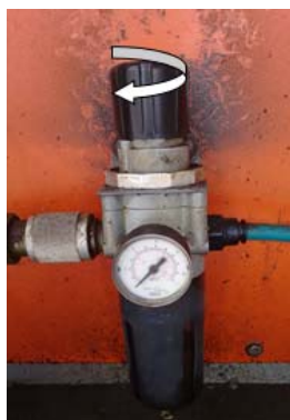
Image 64 – Manometer of the air system
