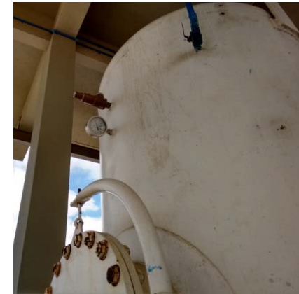
Image 53 - Lung Tank Manometer
