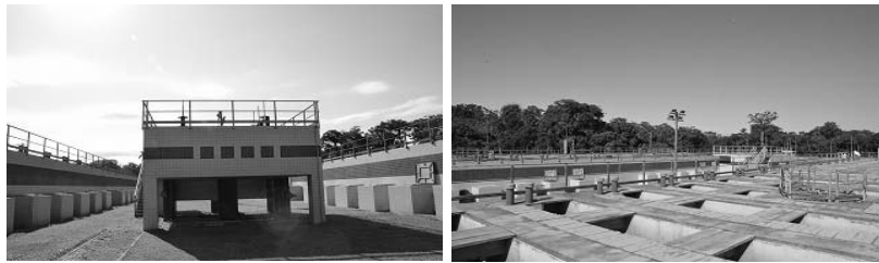
UASB: Six units of UASB
