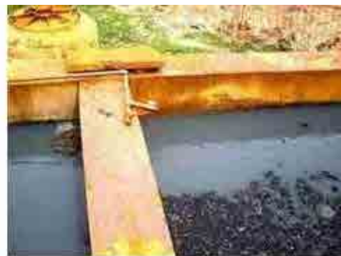
Coagulant dosing pipe (before improved)
