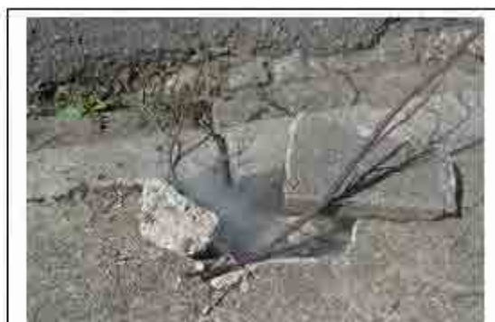
Leakage of smoke from road surface
