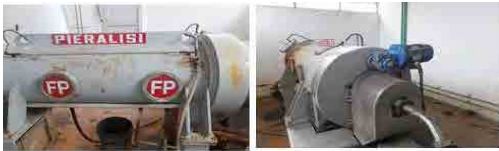
Centrifugal Dewatering Machine in Santa Quiteria STP
