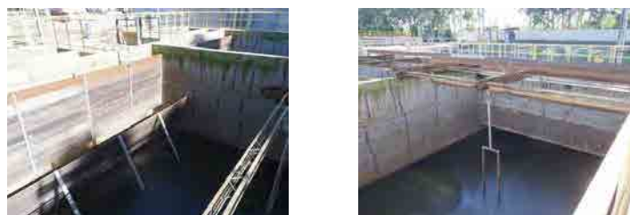
Floatation basin improved in the 3 rd fiscal year (Atuba Sul sewage treatment plant)
