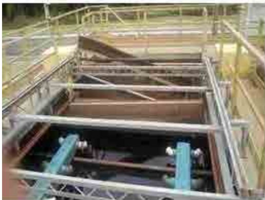
Collector dropped into tank (before improve)
