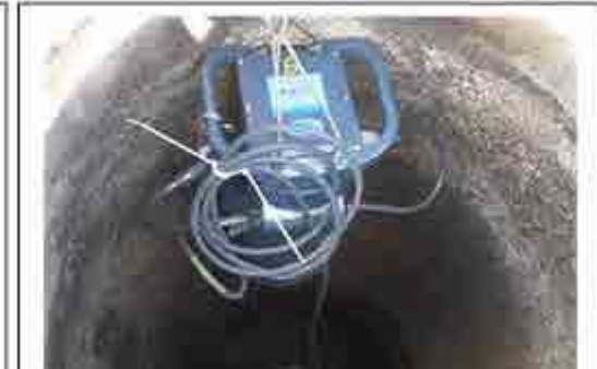
Main body of flowmeter installed in manhole
