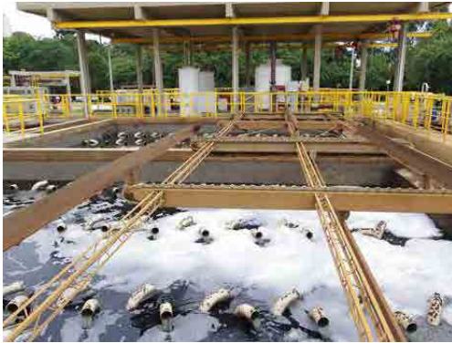
Existing collectors (after improved)
