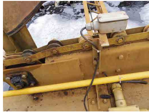
New sensors (after improved)
