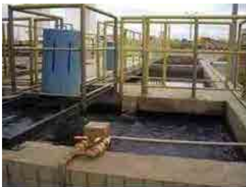
Mixing tank of DAF facility (before improved) (Near side: rapid mixing tank / Far side: floculation tanks)
