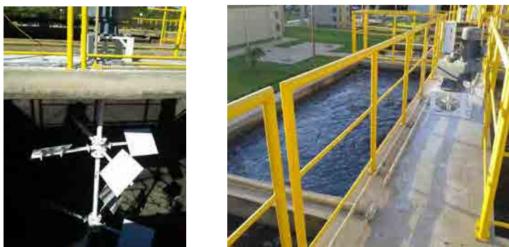
Flocculator installed in the 1 st stage of flocculation basins in the 3 rd fiscal year (after improved)
