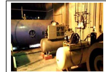
el. Compressor de ar
