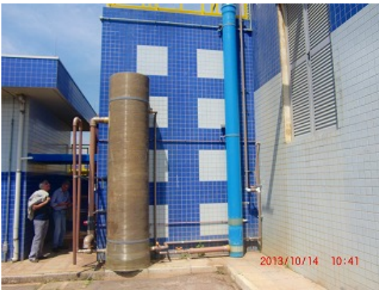
15. Pilot plant of advanced treatment in Irai WTP (right: ozone contacting tank; left: granular activated carbon filter)
