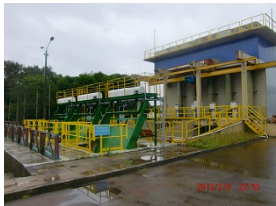
6. Intake of Irai WTP
