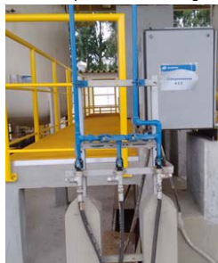
Image 72 - Valves of the compressed air pipeline
