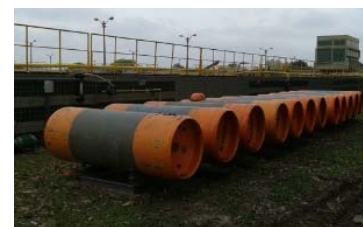
Image 10 - Chlorine Application System
