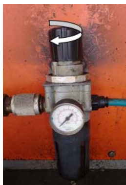
Image 64 – Manometer of the air system
