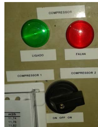
Image 78 - Actuation button of compressors
