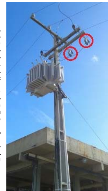
Image 103 - Pole with cutout fuse (floater 01)
