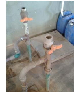
Image 94 - Hatchway of the utilities water well
