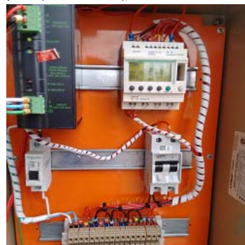
Image 69 - Inside Zelio command panel
