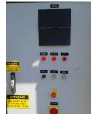
Image 21 – Command panel of automated grates
