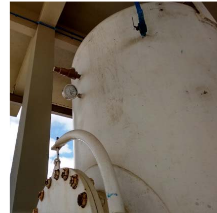
Image 53 - Lung Tank Manometer
