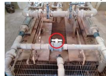
Image 83 - Sludge pipeline valve
