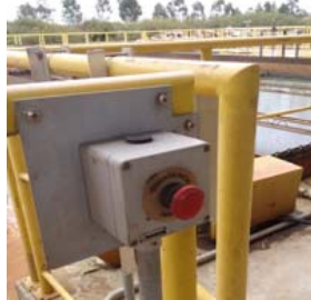
Image 67 - Scraper emergency button
