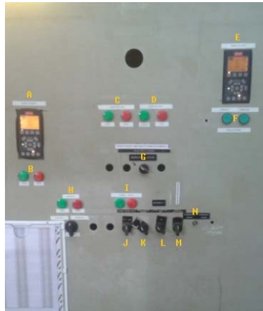
Image 80 – Command panels I and II
