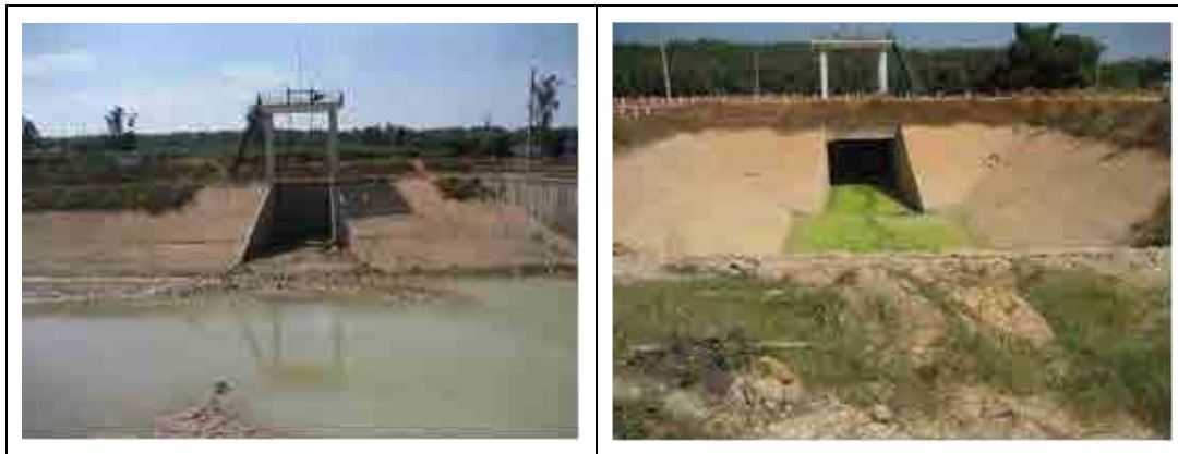
Photo 5.5.1 Existing Intake for New North Binh Duong WTP on Phuoc Hoa - Dau Tieng Canal
