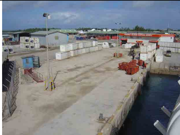
Photo 1-1: Full View of Berth for Inter-island Ferry Berth No. 3 & 4 in Queen Salote Wharf No paving behind the apron area
