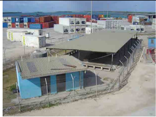
Photo 1-2: Passenger Waiting Shed and Toilet There is no wall for waiting shed, so it is windswept and passengers are suffering from sand dust.
