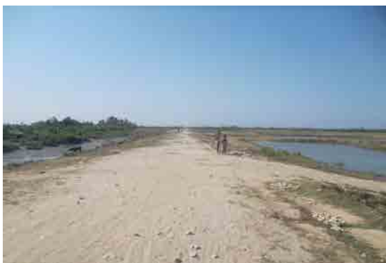
Condition of the road near Hlaingbone Village
