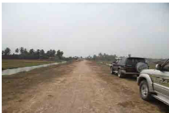
Condition of the road near Tha Kan Bridge
