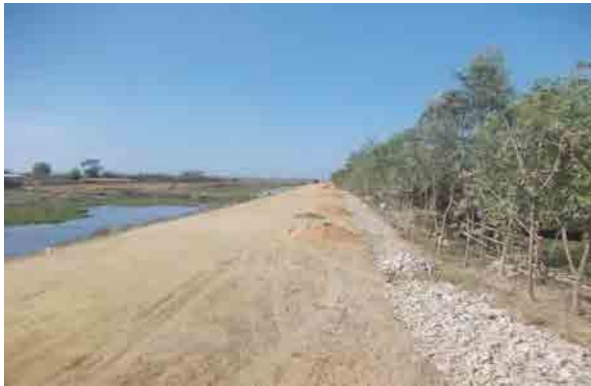
Condition of the road near Zinywellay Village
