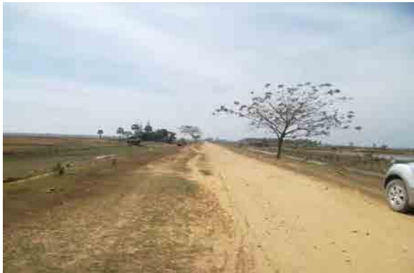
Condition of the road near Dawyein Village
