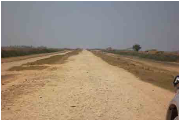
Condition of the road near Kyaonkadun Village
