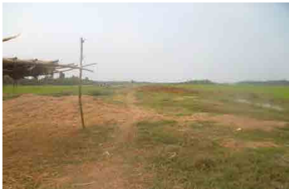
Condition of the road near Ahlalchaung Village
