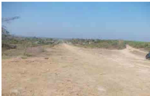
Condition of the road near Ahpyinyesai Village
