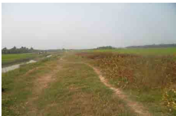
Condition of the road near Kyeechaung Village
