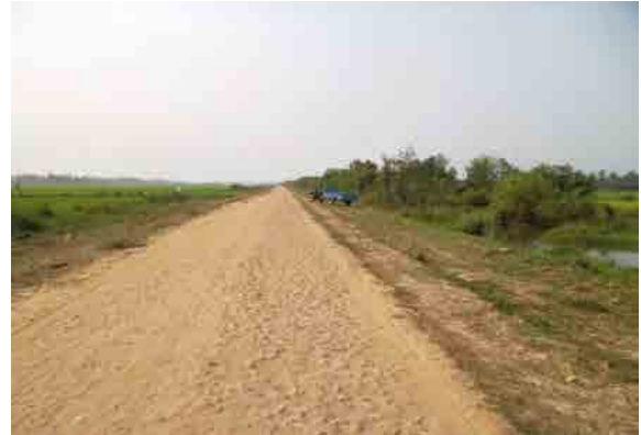
Condition of the road near Nyinaunglay Village
