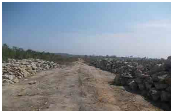
Condition of the road near Ahtwinyesai Village
