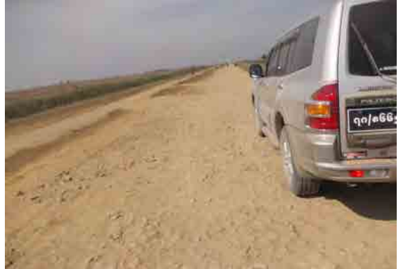
Condition of the road near Phayargone Village
