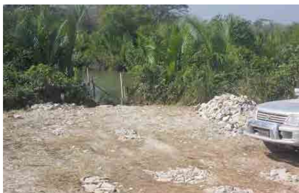
Condition of the road near Ahtwinyesai Village
