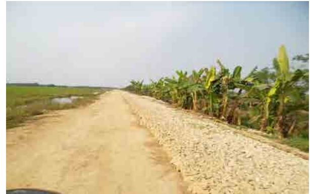
Condition of the road near Penfu Village
