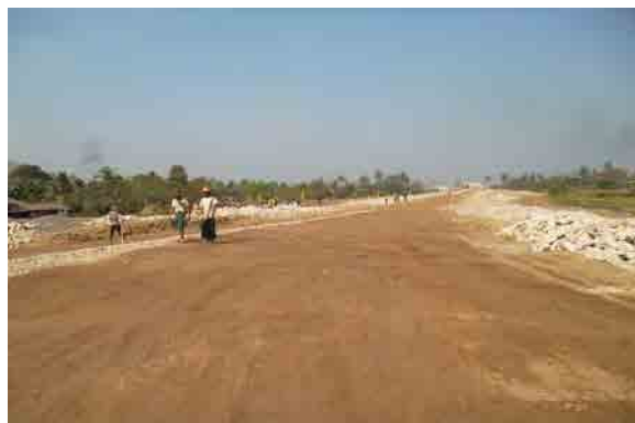
Condition of road at the left bank side of Bogalay Bridge
