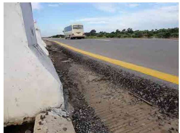
Ph.28 Asphalt overlaying work. Insufficient treatment on the edge. Vibration occurred during even non-heavy vehicle was passing.
