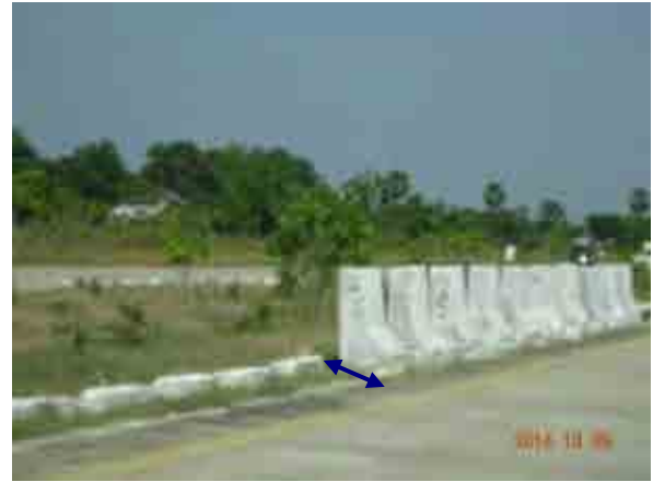
Ph.140 But concrete wall also should be set back.
