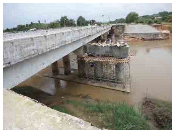
Ph.68 Widening work of the bridge on the opposite side (2-lanes to 3-lanes).
