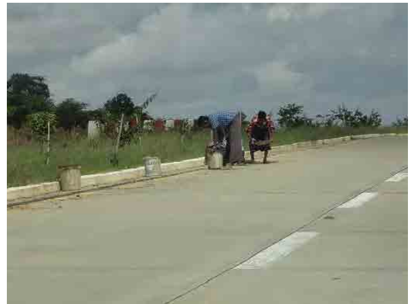
Ph.36 Injection of cement mortal into joint parts between each concrete slabs to prevent water penetration (good example).
