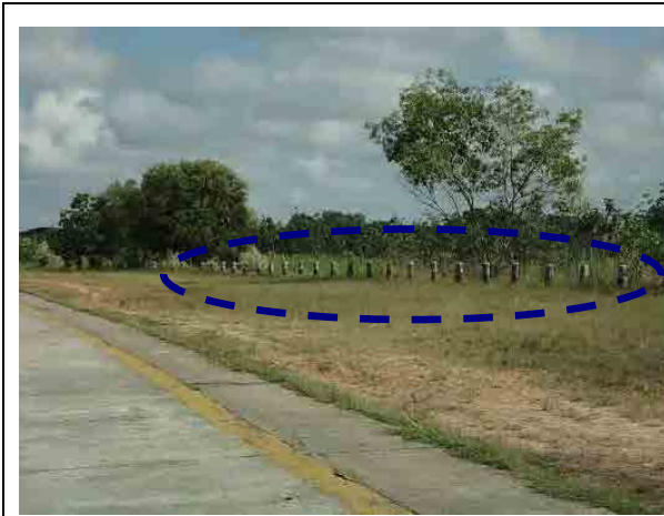
Ph.17 Risk of serious injury on passengers in case of colliding with concrete posts.
