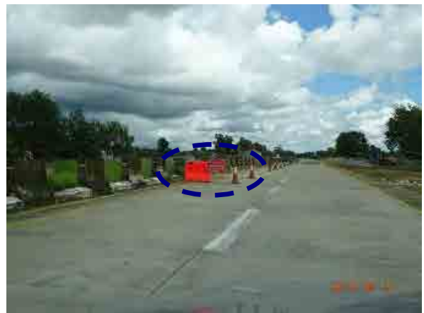
Ph.108 Repair work on median strip. Traffic controlled area should be gradually guided by taper shape.
