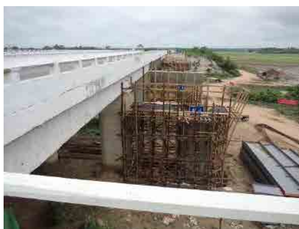
Ph.70 Place of the bus fall accident on May/2015 (198mile). Bridge widening work (2-lanes to 4-lanes) is in progress.
