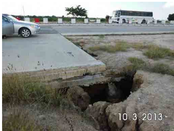
Ph.25 Large cavity under concrete slab. Potential risk of the collapse.
