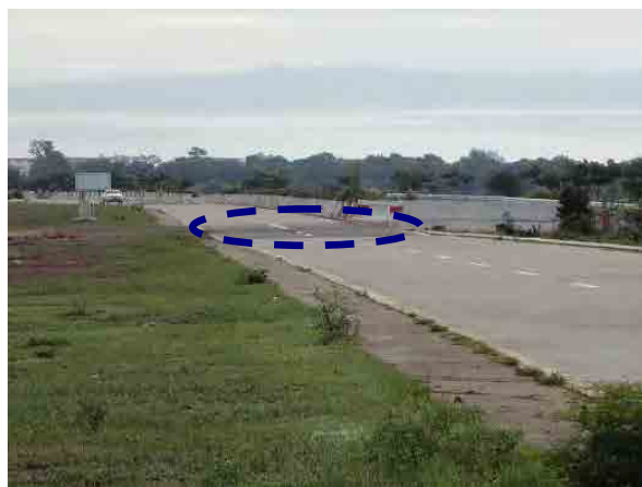
Ph.27 Repair works (asphalt overlaying) on settled parts occurred behind and/or beyond the box culverts.
