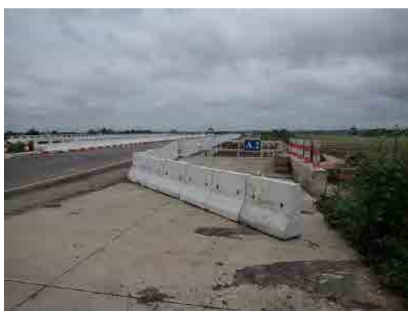
Ph.69 Place of the bus fall accident on May/2015 (198mile). Bridge construction site.
