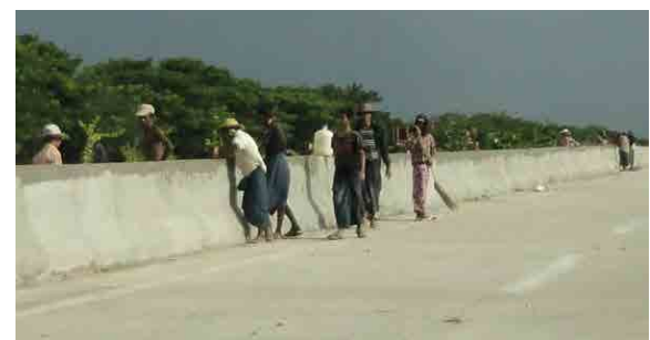
Ph.40 Workers took a rest within carriageway (prohibited work manner).
