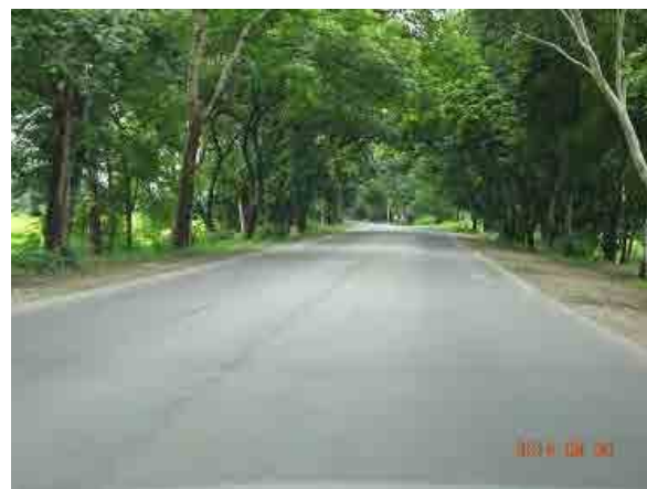
Ph.82 Road condition was good in general. But lane mark should be painted to divide traffic flow clearly.
