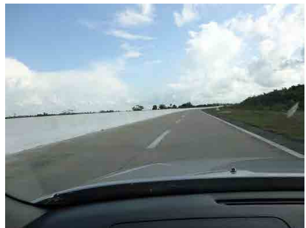
Ph.38 Continuous concrete wall on median strip side instead of concrete block (good example). Overrun will be prevented.
