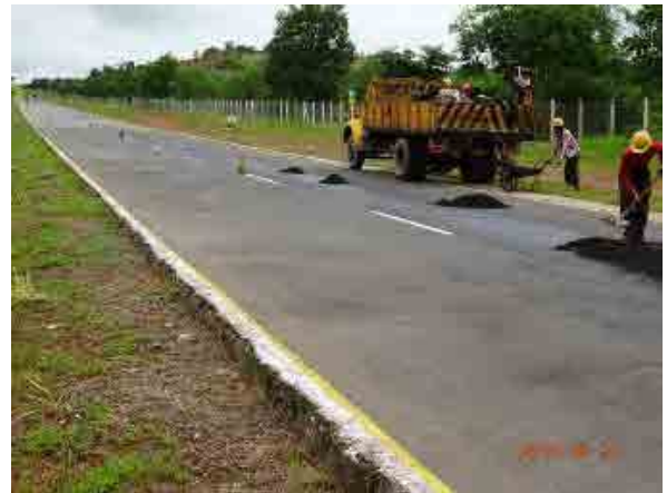
Ph.106 Repair work. Work area was clearly surrounded by the cones (good example).
