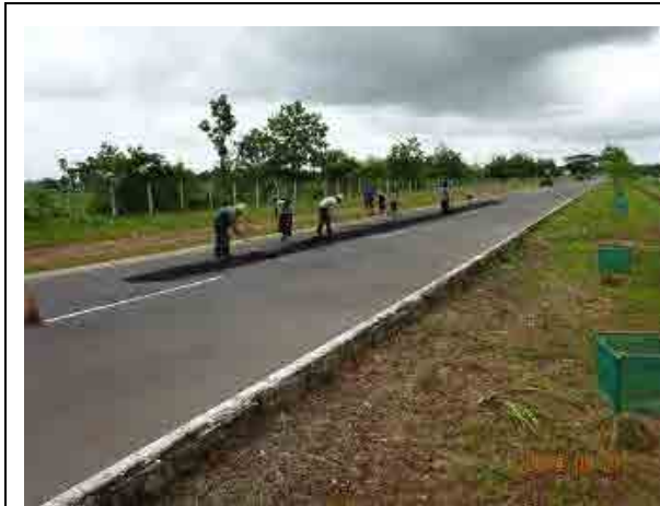
Ph.105 Repair work. Work area was clearly surrounded by the cones (good example).
