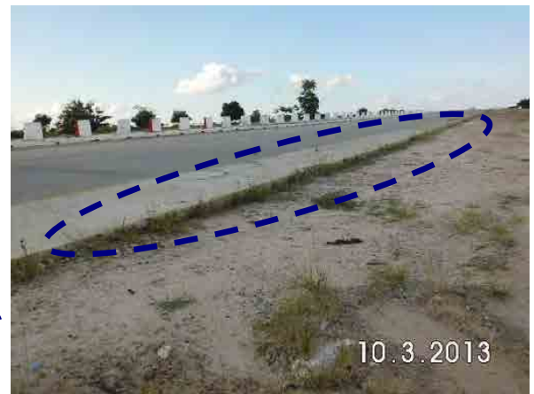
Ph.24 Gap occurred between shoulder and the outer area (photo from behind direction).
