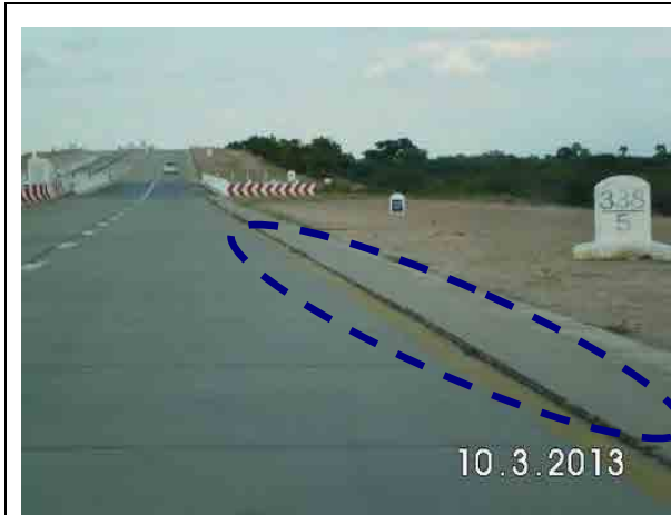
Ph.23 Gap occurred between carriageway and shoulder.
