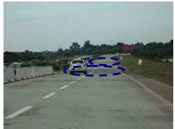
Ph.26 Repair works (asphalt overlaying) on settled parts occurred behind and/or beyond the box culverts.
