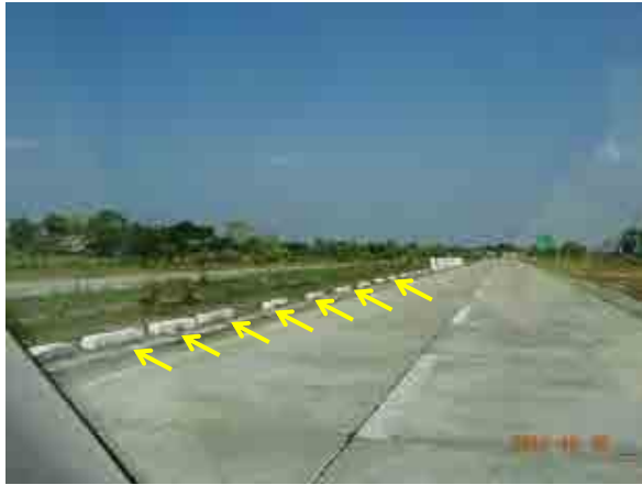
Ph.139 Concrete curb was set back to median strip side to secure shoulder width (good action).
