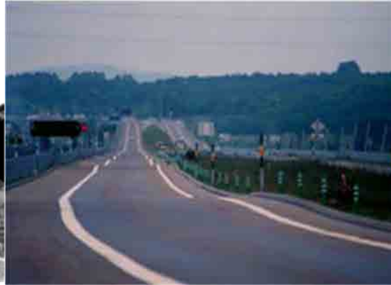
Figure 1-10 Example of settlement on road surface 4)
