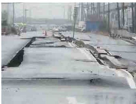
Figure 1-14 Road surface deformation due to liquefaction 5)
