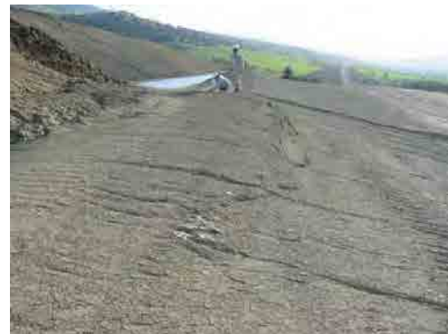
Figure 1-6 Swelling caused by slip failure (TCP)
