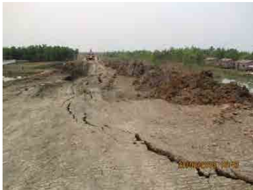
Figure 1-5 Clacks and depression caused by slip failure (Myanmar)
