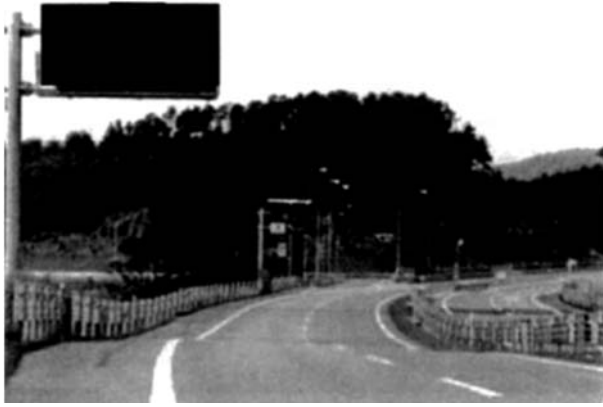
Figure 1-9 Example of settlement on road surface
