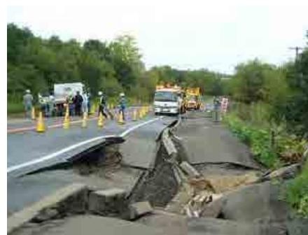
Figure 1-15 Road collapse due to earthquake 6)
