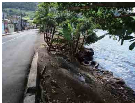
Location 3: Road Elevation MSL+3.0m
