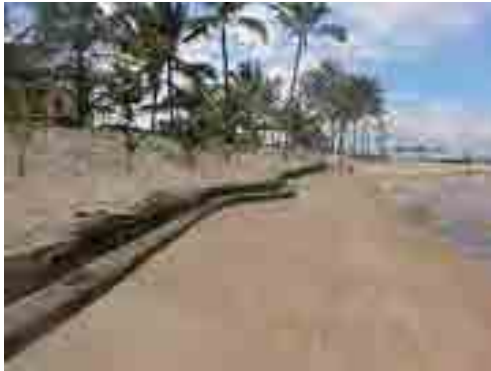
Photo A: Beach and Revetment in front of the Hotel at the East
