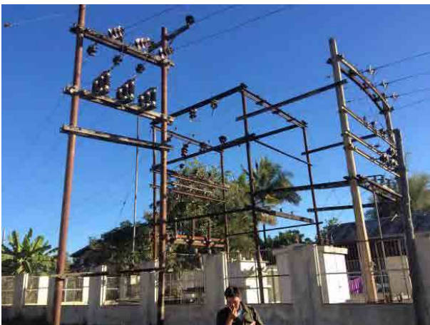
Mai lone Substation (33/11kV, 1MVA)
