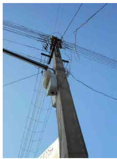
0.4kV Distribution Line near Market
