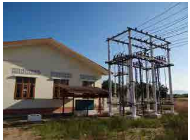
Industrial park building and 11kV feeders
