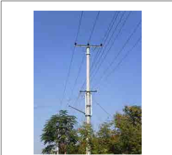
11kV & 400V distribution line
