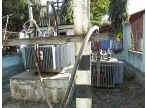
Distribution Transformer (315kVA×2)
