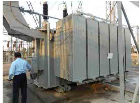
Pyay Substation Transformer No.2
