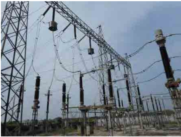
230kV/33kV Kamanut Substation
