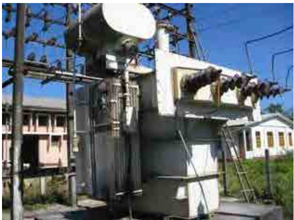
66/6.6kV 2 MVA, Myaing gale SS
