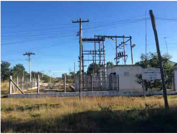
500 Acre Substation (33/11kV, 5MVA)
