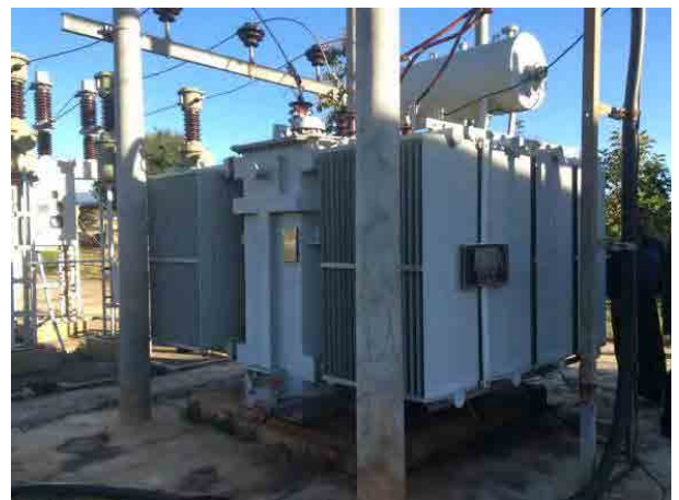
Yawar tan Shae SS 5MVA Transformer
