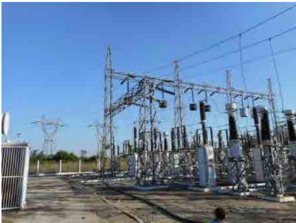
Makyikan Substation (MEPE) (132/33kV 15MVA×1, 132/33/11kV 60MVA)
