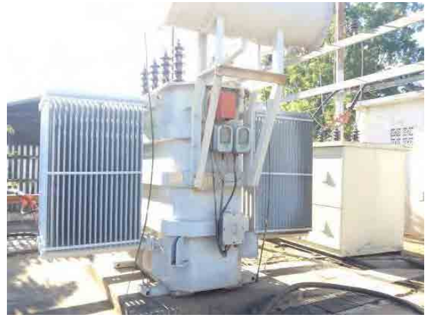
500 Acre SS 5MVA Transformer
