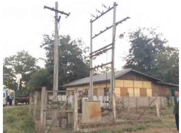
11/0.4kV Transformer in Loikaw city
