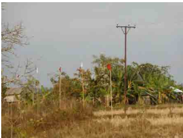
11kV line to Wettigan
