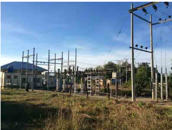
Yawar Tan Shae Substation (33/11kV, 5MVA)
