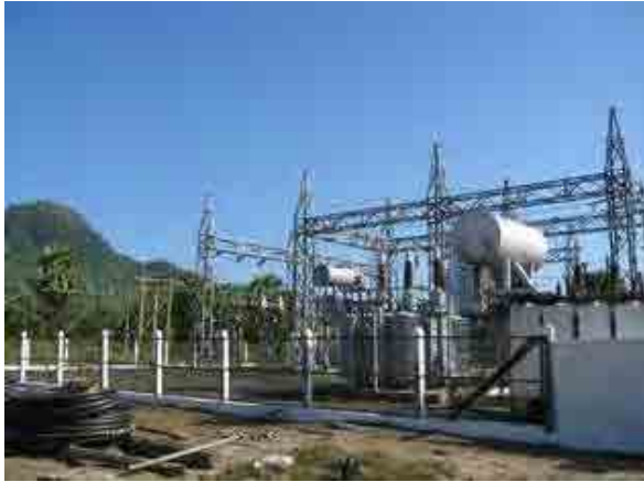
66/11kV 10MVA x 2, Hpa-An main SS
