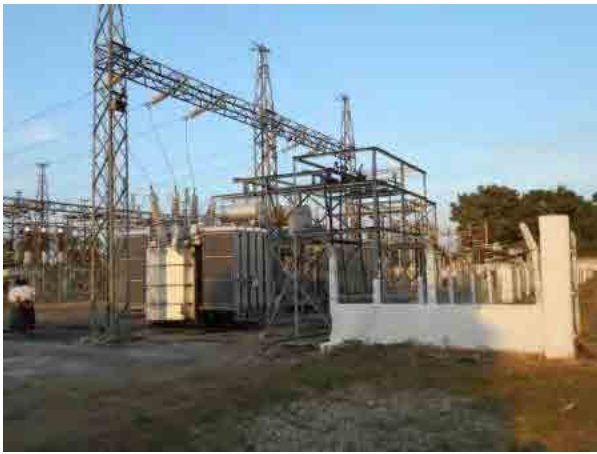
66kV/11kV Pyay Substation
