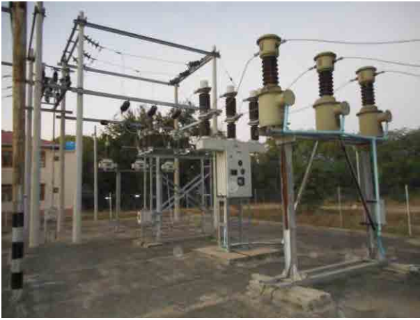
Minbu Substation (33/11kV 5MVA)
