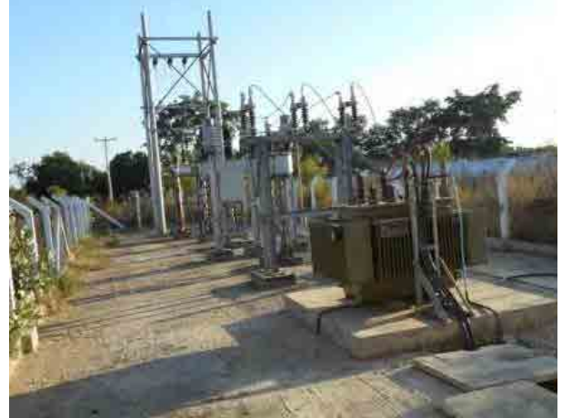
Hluttaw Substation (33/11kV 1MVA×1)
