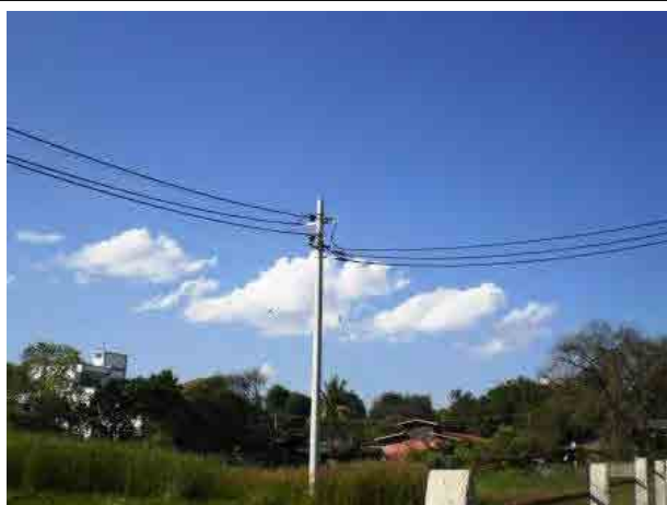
33/11kV Chi Pa SS 33kV Transmission Line
