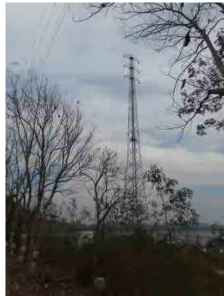
Steel Tower for 66kV Line over Ayeyarwady River
