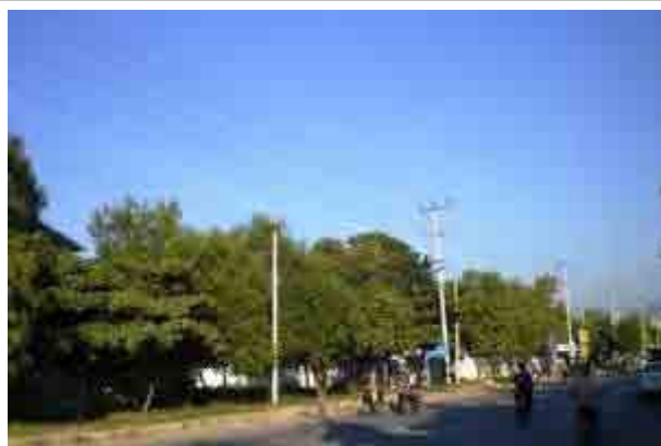
33kV Distribution line (Upper circuit, Concrete pole, 1cct)
