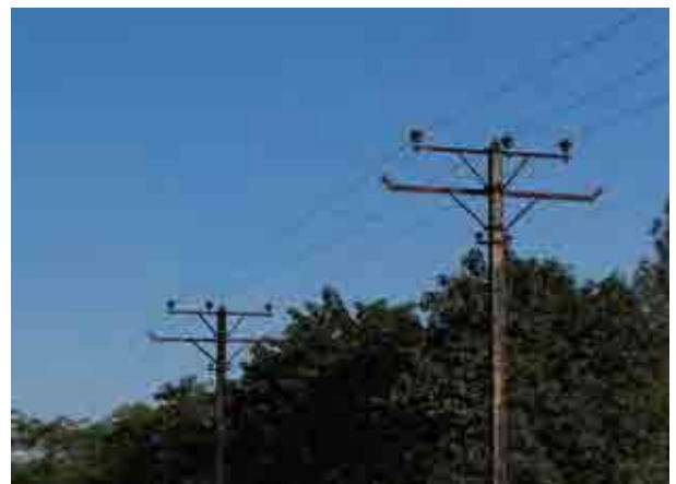
MV Distribution line with
