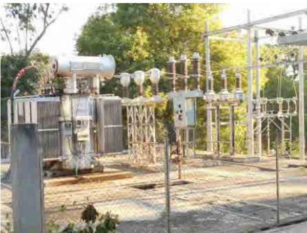
Natmauk Substation (33/11kV 10MVA×1)
