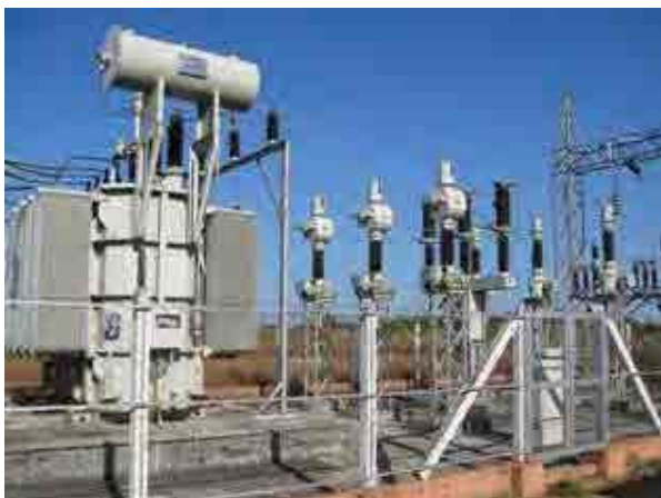
66/11kV 20MVA, Industrial Park SS
