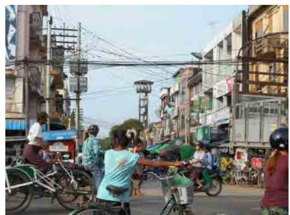
11kV and 0.4kV distribution line
