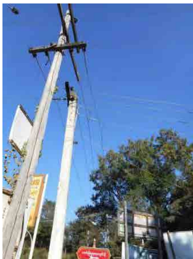
Cracked wooden pole
