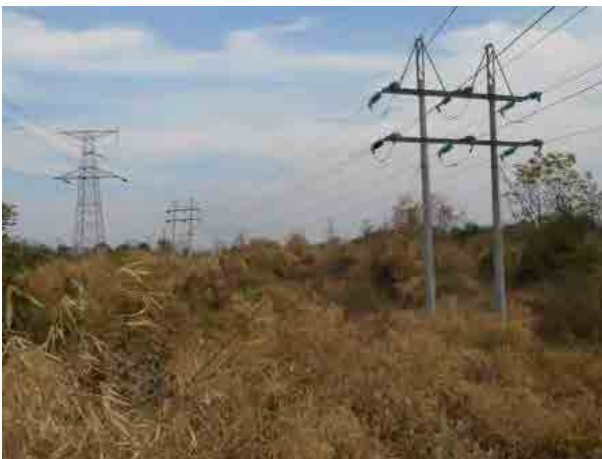
132kV Line and 66kV Line
