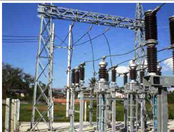
33/11kV Chi Pa SS (10MVA×1No.)
