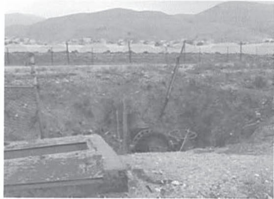
A Turnout Structure from the Main Canal at Middle Jordan Valley Irrigation Scheme
