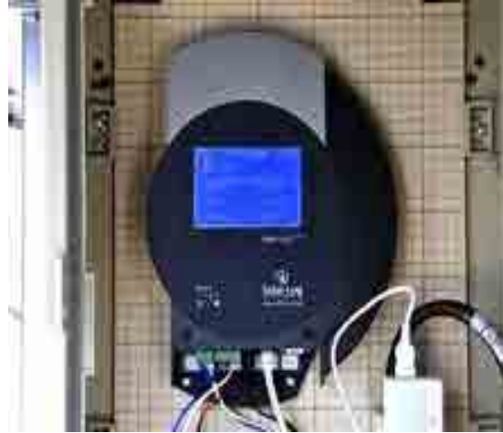
Source: Next Energy & Resources Co., Ltd. http://www.nextenergy.jp/service/mega_solar.php
