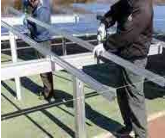
Source: Next Energy & Resources Co., Ltd. http://www.nextenergy.jp/service/mega_solar.php
