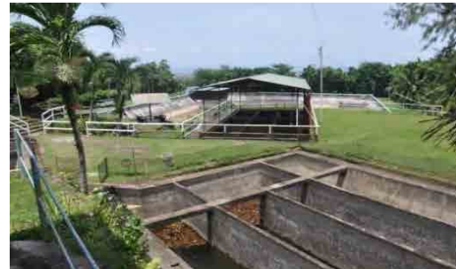
Tisa Water Treatment Plant
