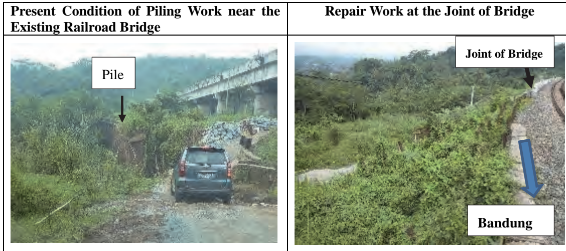
Figure 4.2-9 Condition of Existing Landslide (Sta. 81km)
