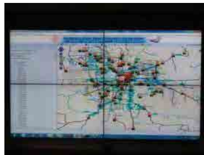
Video Wall at Control Station
