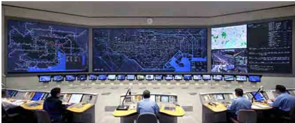
Figure 2.87 Example of Traffic Control Centre
