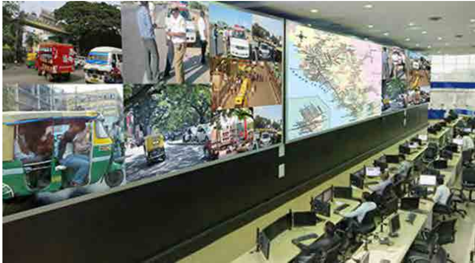
Figure 2.38 Video Wall at Traffic Management Centre of Bangalore Traffic Police
