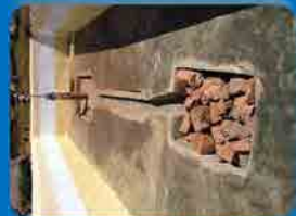
Soak-pit and Floor
