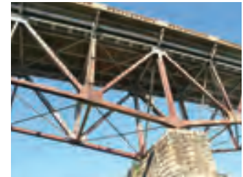
Rusted truss members of the Old Bridge
