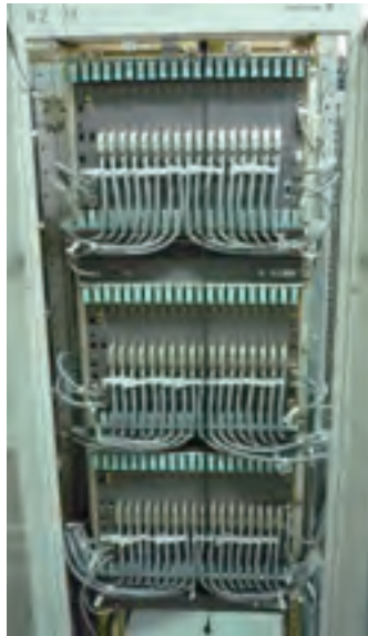
Digital Switching System
