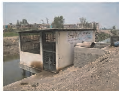
Reuse Pump Station
