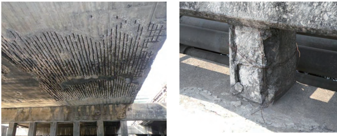
Figure 74 Site Photos of Damage Shown in the Database
