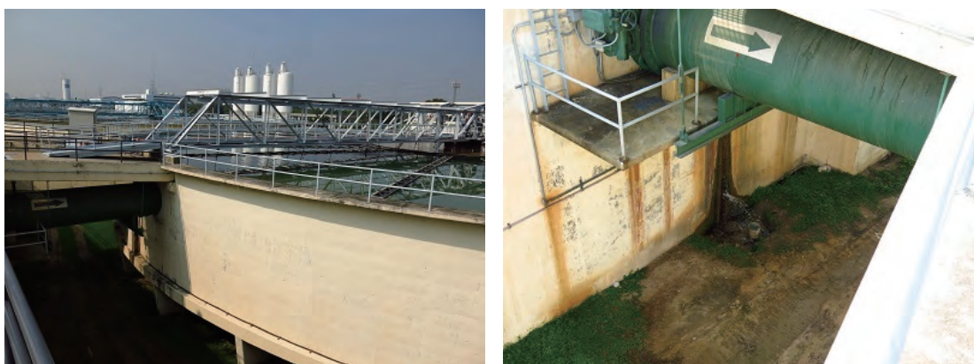
Figure 84 Water Leakage in Water Purification Facility
