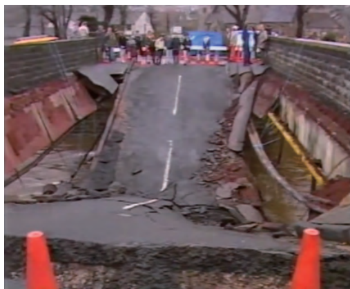
Figure 30 Collapse of a Bridge Caused by Breaks of Pre-stressing Steel Bars 25
