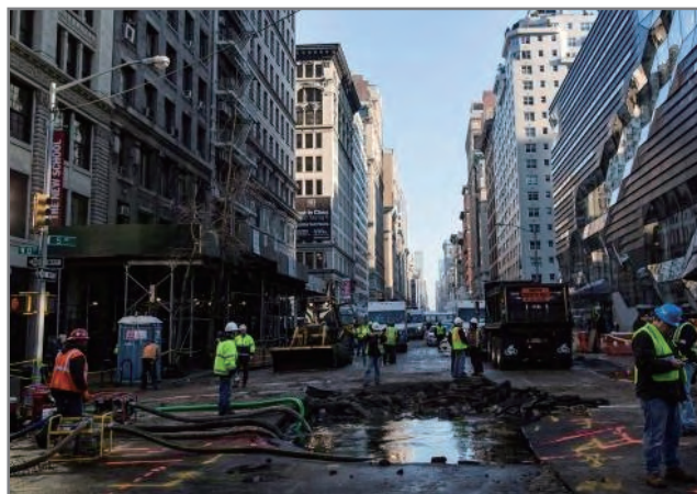
Figure 26 Road Caved in due to the Water Main Break (January 15, 2014) 19
