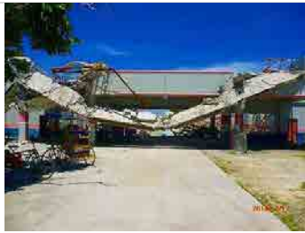
Photo 23. This photo is The gymnasium at Guiuan city. This building collapsed by strong wind.
