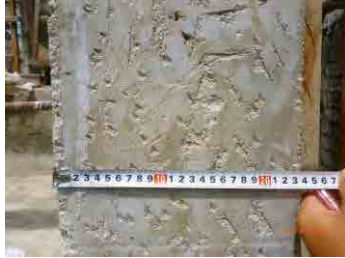
Photo 21. This is chipping surface of concrete column of small private building. This chipping is for mortar apply.
