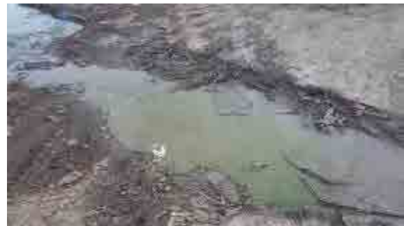
Dirty Water Deposit at Yard-1
