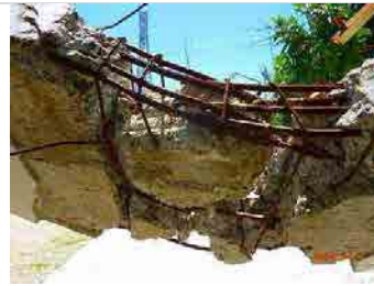
Photo 24. This photo is center of collapsed beam : The splice of re-bar at photo upper part is bottom of beam center. This splice place was prohibited.
