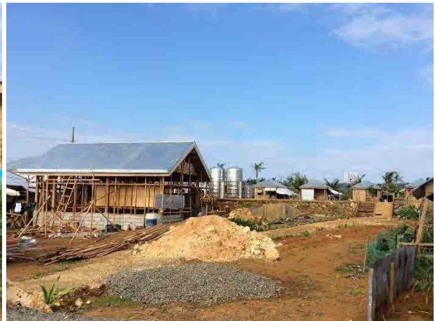
Figure 9.5-30 Water Supply Facility and a Community Facility in the Temporary Shelter Site
