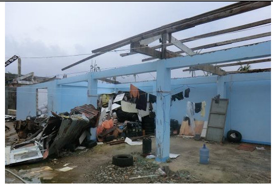
Damaged Nursery Facilities
