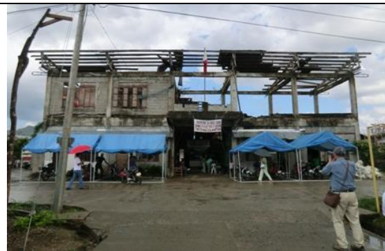
Damaged office due to aging and by typhoon (Lawaan)
