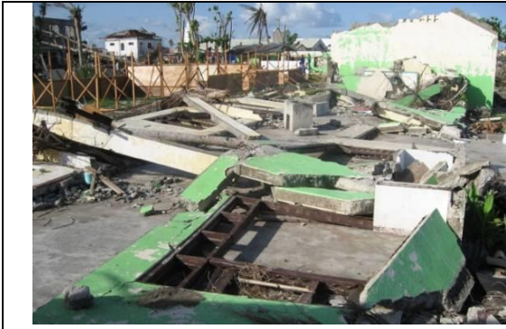
Collapsed Elementary School
