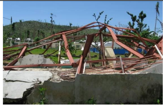
Collapsed School of Steel Construction
