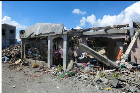
Collapse and Derelict Building
