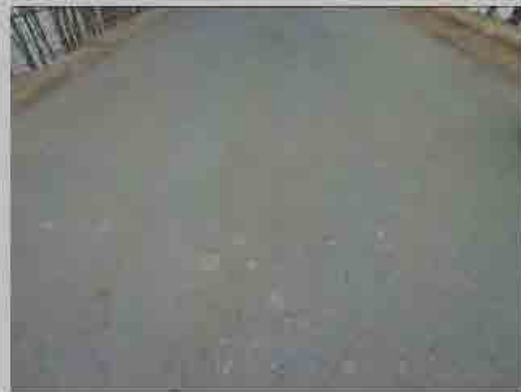
No. 4 Condition of road surface
