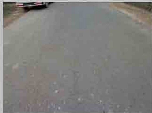
No. 4 Condition of road surface
