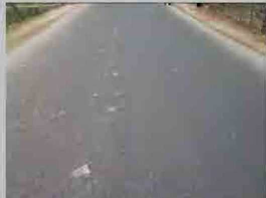
No. 4 Condition of road surface
