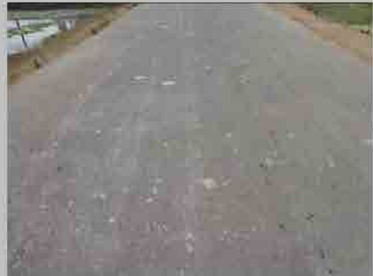
No. 4 Condition of road surface
