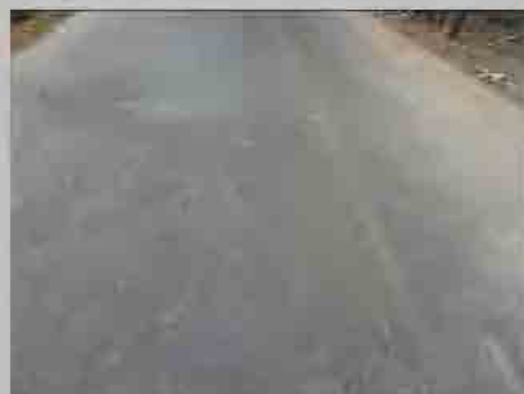
No. 4 Condition of road surface
