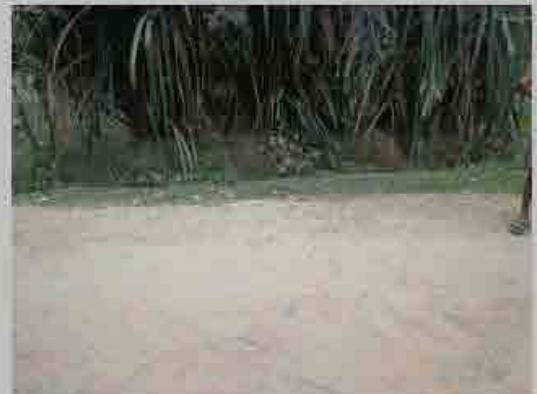
No. 4 Condition of road surface
