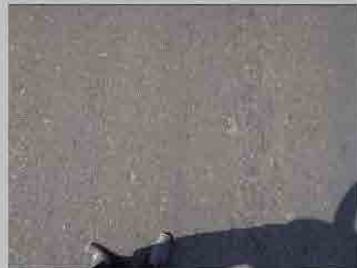
No. 4 Condition of road surface
