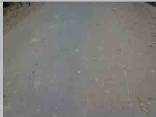
No. 4 Condition of road surface
