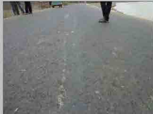
No. 4 Condition of road surface
