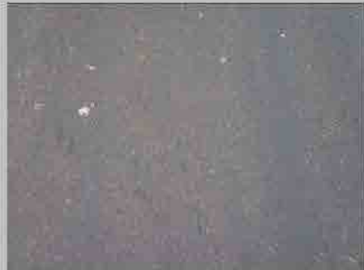
No. 4 Condition of road surface
