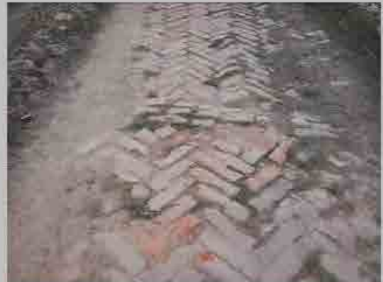
No. 4 Condition of road surface
