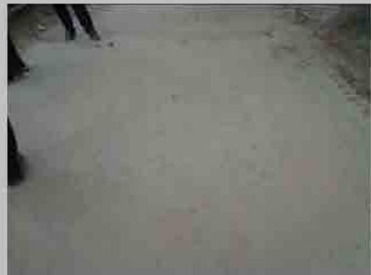
No. 4 Condition of road surface
