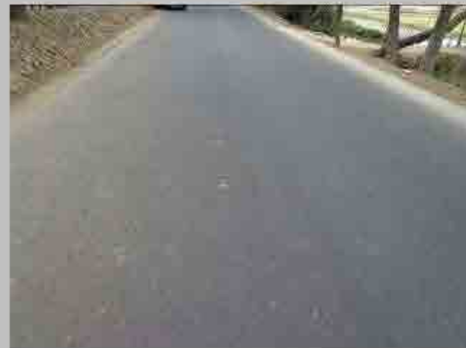
No. 4 Condition of road surface
