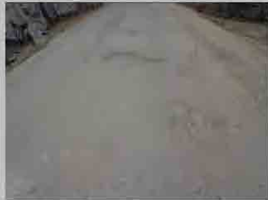
No. 4 Condition of road surface
