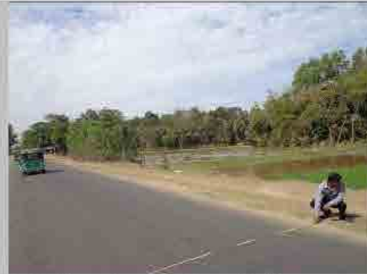
No. 2 Distance view to the forward right
