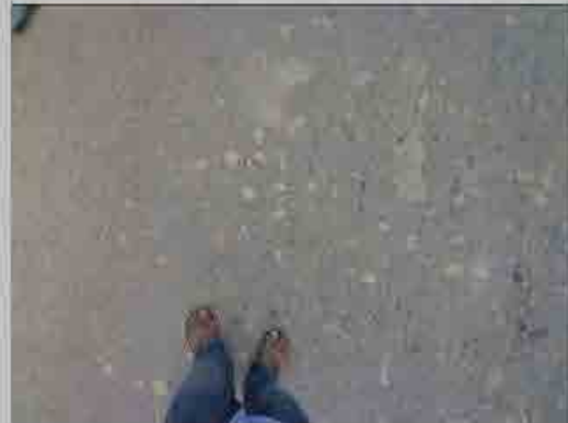
No. 4 Condition of road surface
