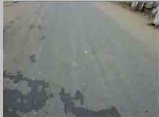
No. 4 Condition of road surface
