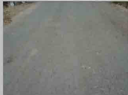
No. 4 Condition of road surface
