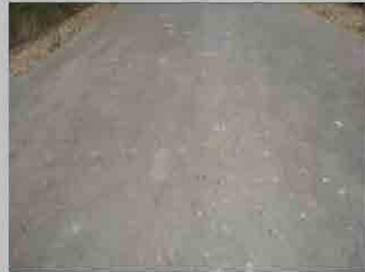
No. 4 Condition of road surface
