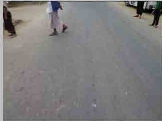
No. 4 Condition of road surface
