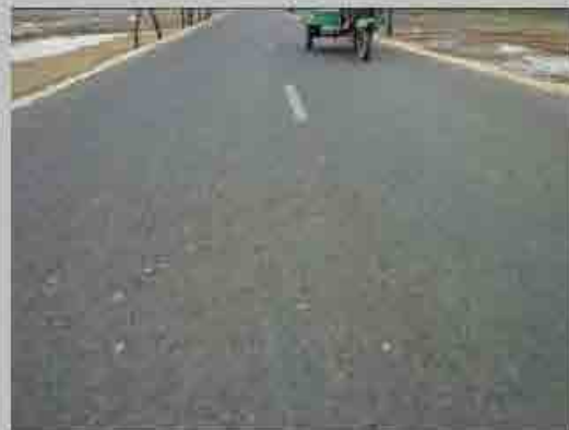
No. 4 Condition of road surface
