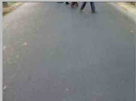
No. 4 Condition of road surface
