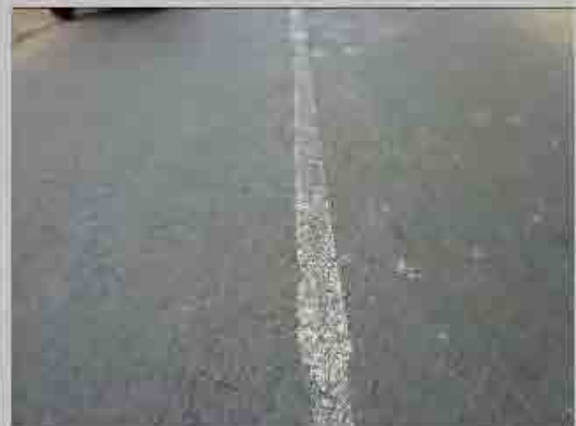
No. 4 Condition of road surface
