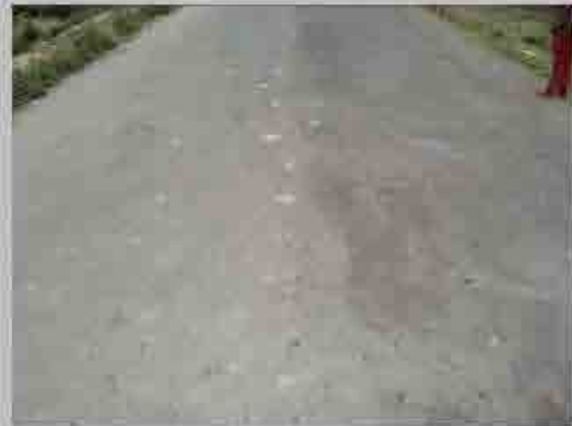
No. 4 Condition of road surface:
