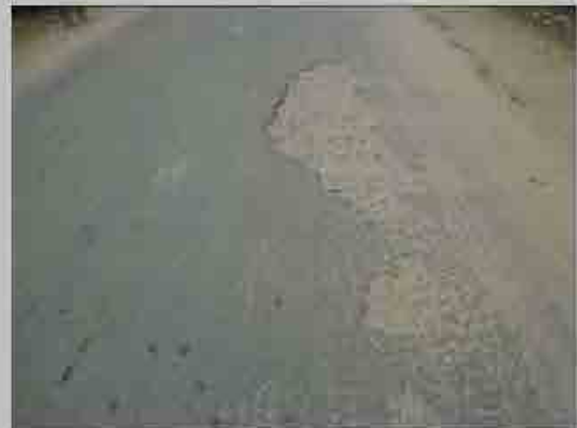
No. 4 Condition of road surface
