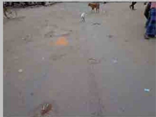
No. 4 Condition of road surface
