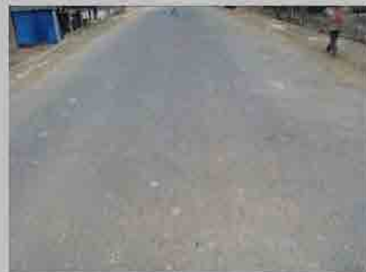
No. 4 Condition of road surface
