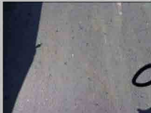
No. 4 Condition of road surface
