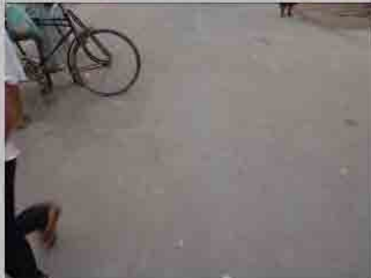
No. 4 Condition of road surface
