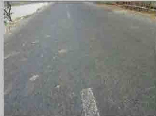
No. 4 Condition of road surface
