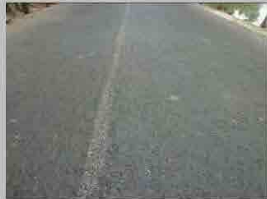
No. 4 Condition of road surface
