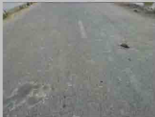
No. 4 Condition of road surface
