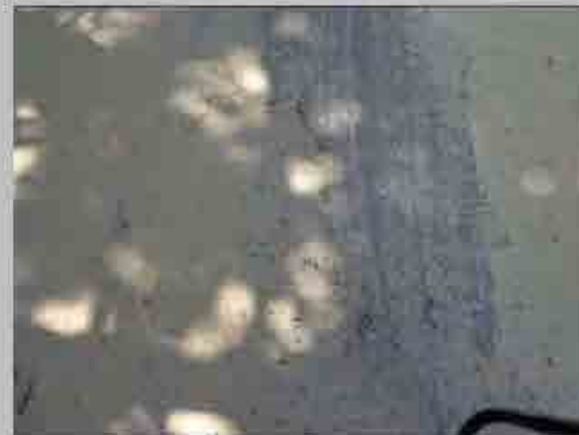
No. 4 Condition of road surface
