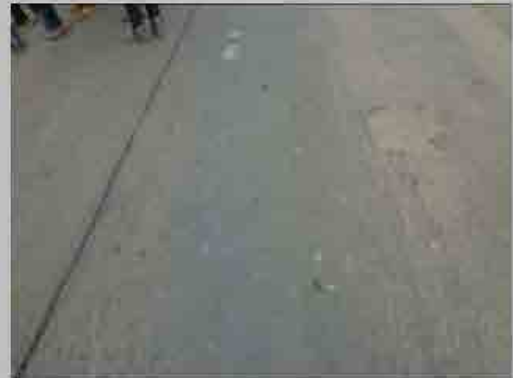
No. 4 Condition of road surface
