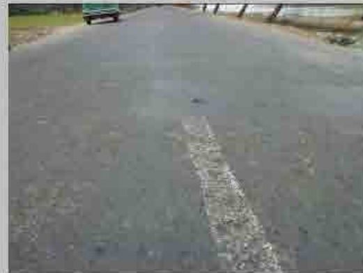
No. 4 Condition of road surface
