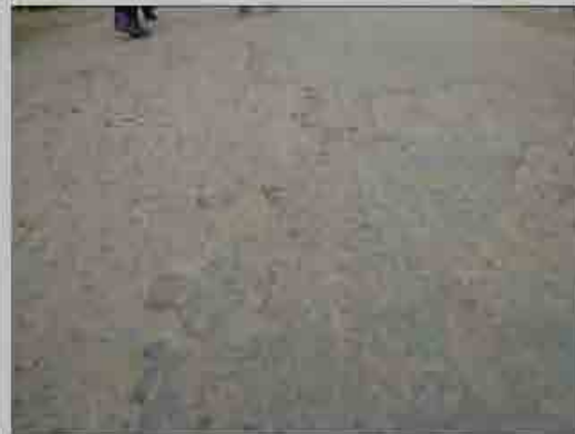
No. 4 Condition of road surface
