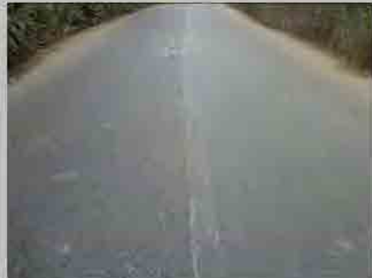
No. 4 Condition of road surface
