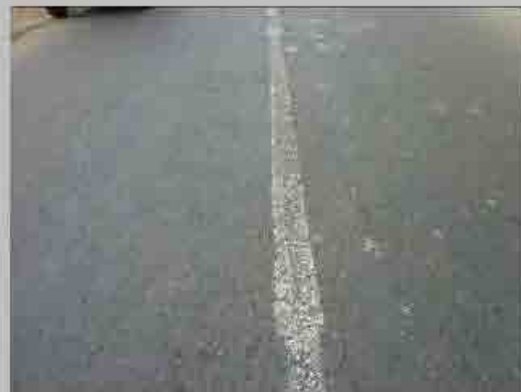
No. 4 Condition of road surface
