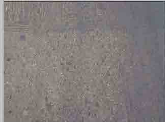
No. 4 Condition of road surface
