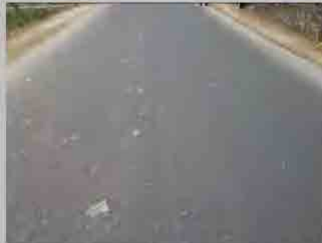
No. 4 Condition of road surface
