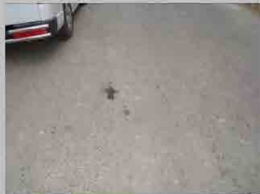
No. 4 Condition of road surface
