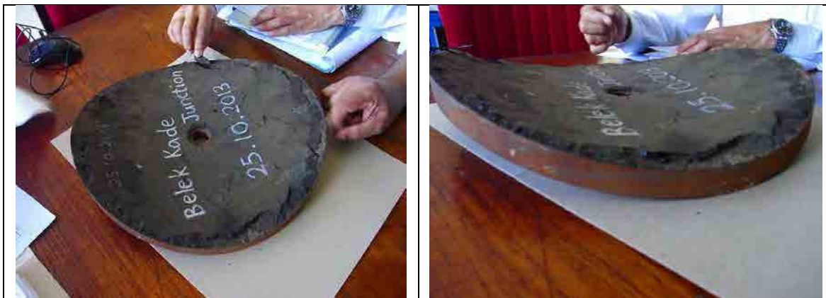
Photo 5.2.1: Photos for Cut Piece of 800 mm Diameter of Old CI Pipe
