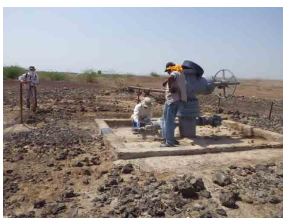
Opening the valve of TD-6
