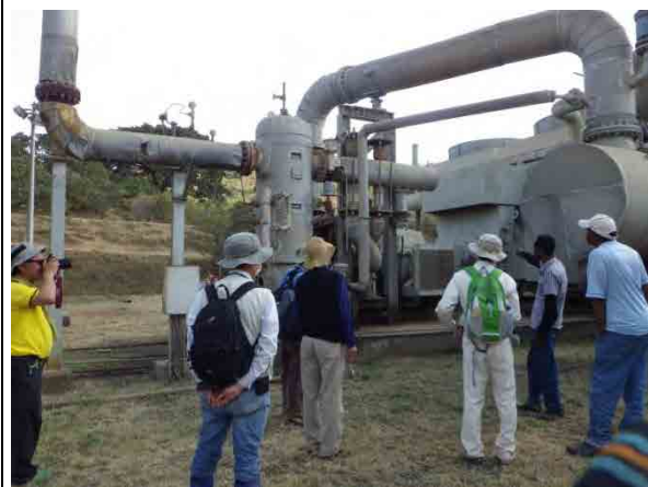
Turbine and Generator in Aluto-Langano Geothermal Power Plant
