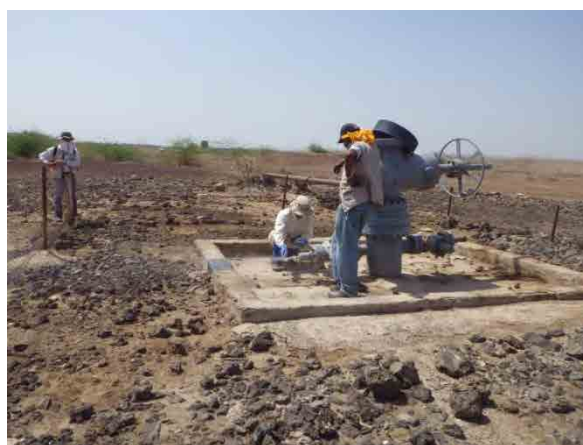
Opening the valve of TD-6
