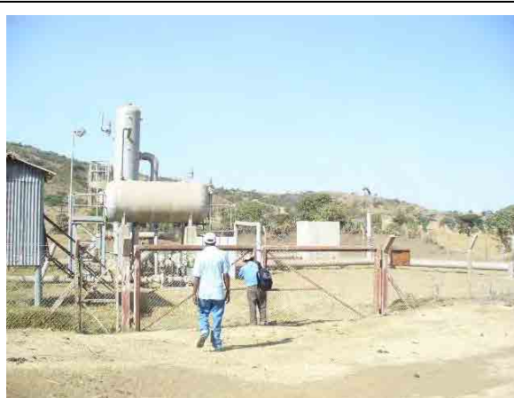
Geothermal well and separator in LA-4
