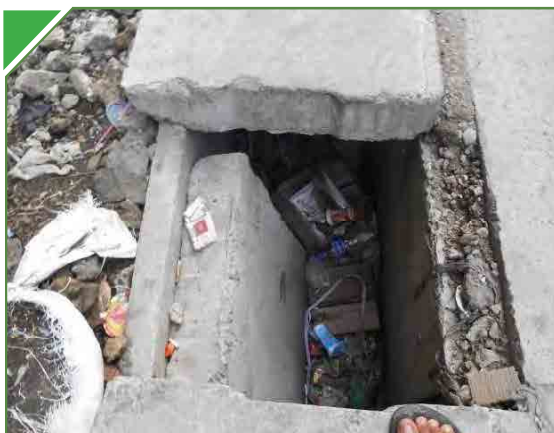
Failed Cover at Kebonpala 1
