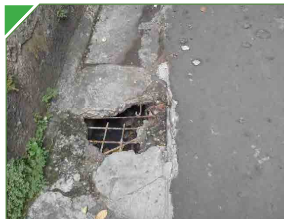
Failed Cover KS Tubun
