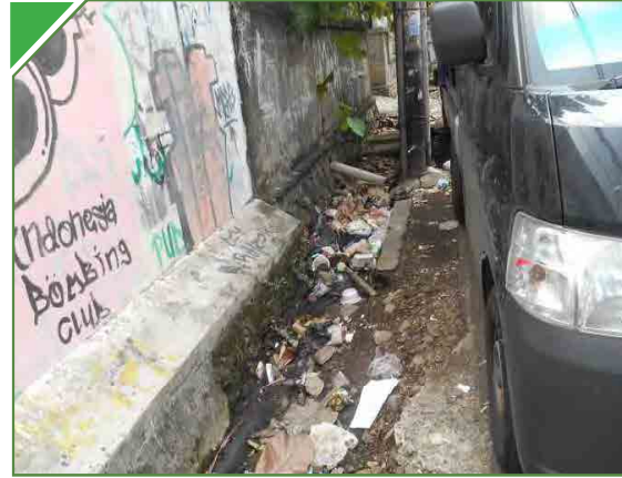
Clogging at Jl. Kebonpala 2
