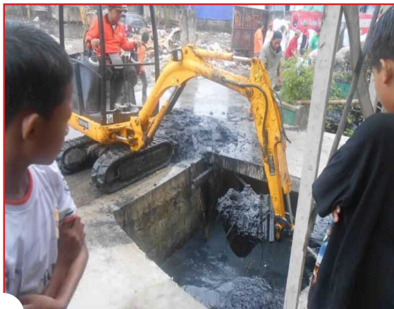
Excavation of sedimentation by mini bac khoe at PHB Klingkit Rawa Buaya - Cengkareng
