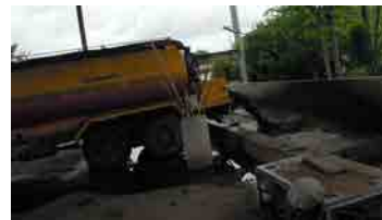
Receiving Screen & Tank
