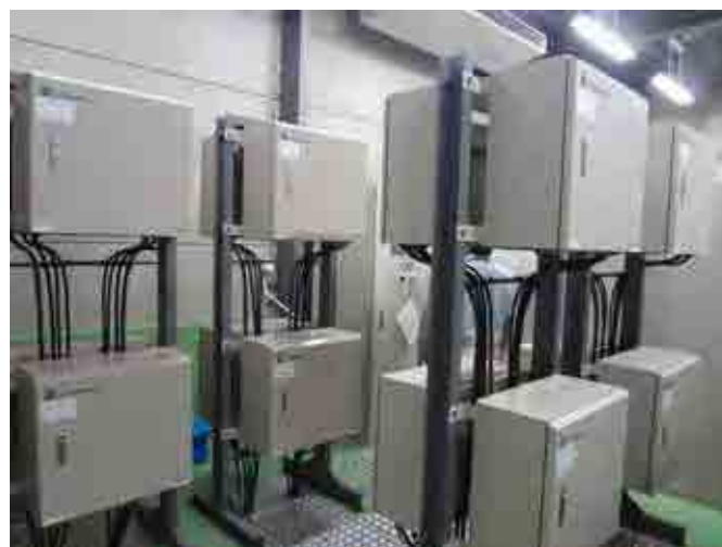
Figure 1-5 Example of a PV System with Commercialized PCS in the Remote Islands of Okinawa
