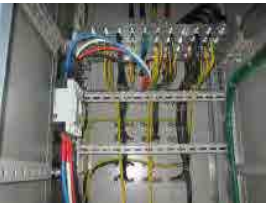
(AC STATION DISTRIBUTION PANEL) (F12)
