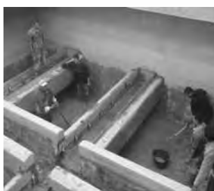
ADJUSTING FILTERS SAND LEVEL
