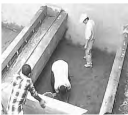
ADJUSTING FILTERS SAND LEVEL
