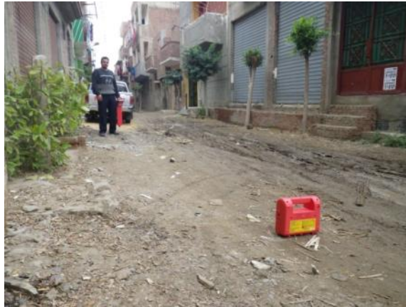
Figure 4.2-17 Training of Metal Pipe Locator on MCWW
