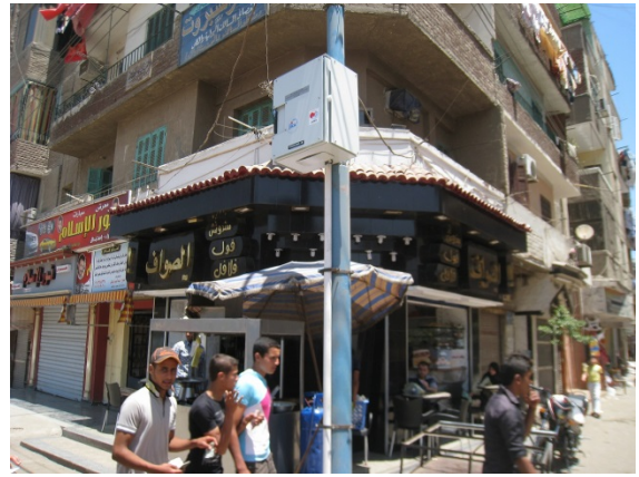
Installation of telemeter at street side for data transfer, May 2013
