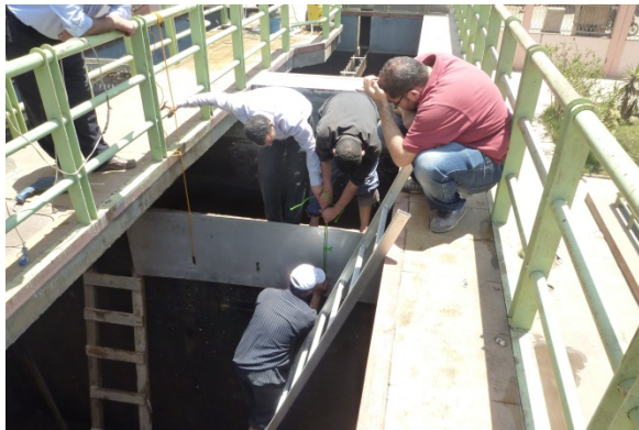
Improvement activity of filter runtime (adjustment of weir level in sedimentation tank) at Gezy IMRP in MCWW, May 2013
