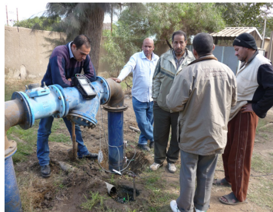
Check amount of flow meter of NWR team of MCWW, Ashama well station, December 2012
