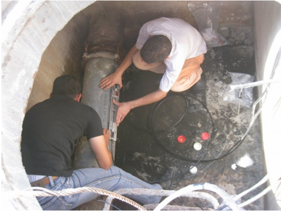
Installation of water flow meter in chamber for water flow monitoring, May 2013
