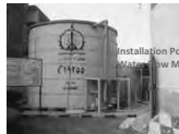
1 Raw Water Flow Meter Availability: Available Location: Before Aeration & Sedimentation Tank Pipe Dia.: Not Confirmed Chamber Size: Not Necessary
