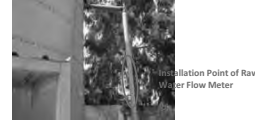
1 Raw Water Flow Meter Availability: Available Location: Before Aeration & Sedimentation Tank Pipe Dia. : 150mm (PVC) Chamber Size: Not Necessary
