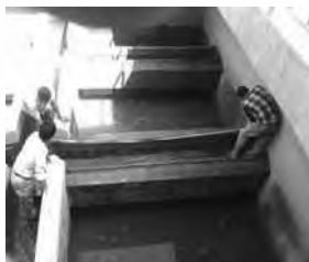
ADJUSTING WEIR LEVEL
