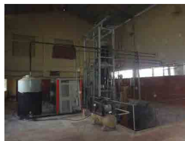
Source: JICA Survey Team Aromatic Oil Extraction Plant (Naga Fragrance Pvt. Ltd.)
