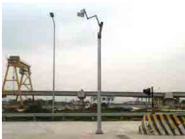
ETC Antenna (Cau Gie – Ninh Binh)
