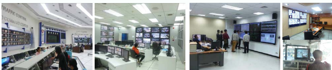
Thailand: Traffic Control Center, CCTV Monitoring Center, Expressway Control Center
