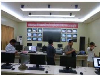
Laos: CCTV Monitoring Center (By Police)
