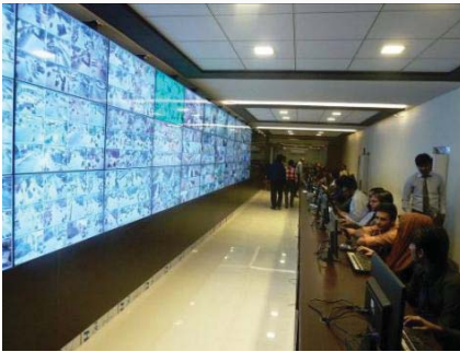
Command & Control Center (KMC)
