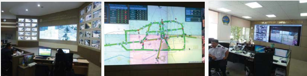
Mongolia: Traffic Control Center, CCTV Monitoring by Police
