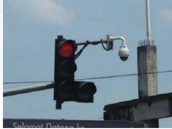
Traffic Signal & CCTV (Malaysia)
