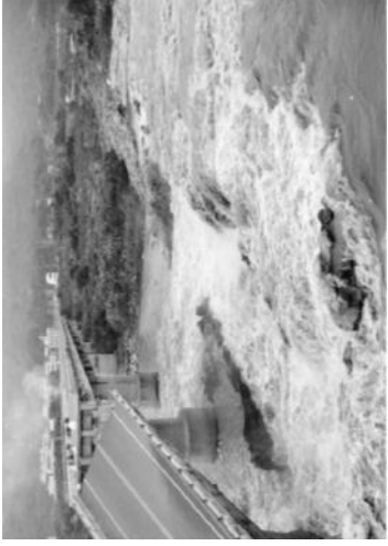
Surface rupture in 1999 Taiwan, Chi-Chi earthquake (Taken by Prof. Abe, the University of Tokyo)
