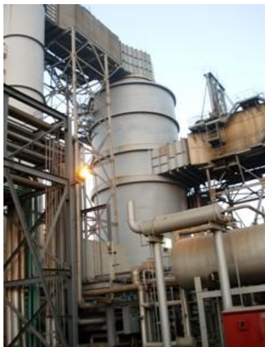
Photo 6-5 Flue gas de-sulfurization system
