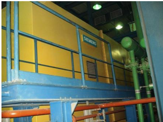
Photo 4-3 Gas turbine generator
