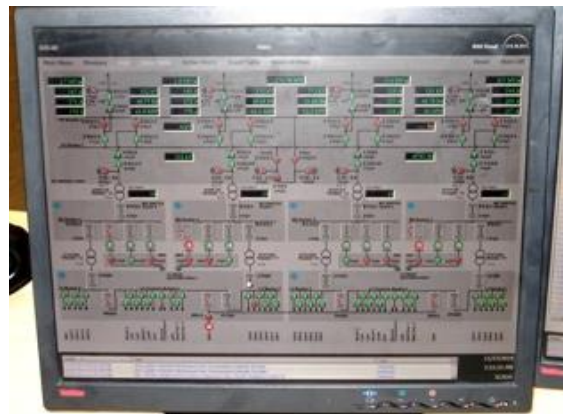
Photo 7-4 Operation monitoring system screen 2
