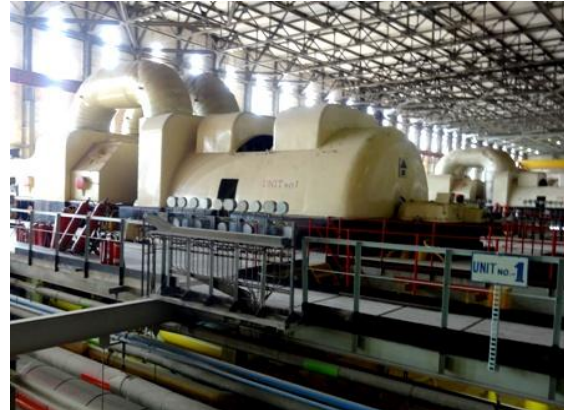
Photo 2-2 Unit no.1 turbine generator
