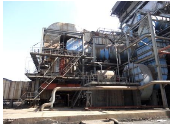
Photo 2-4 Exhaust gas duct
