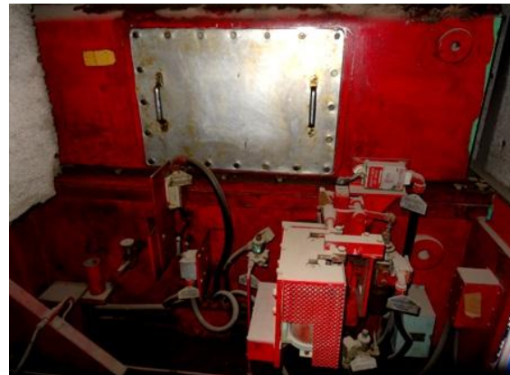
Photo 1-4 No.1 Turbine protection switches
