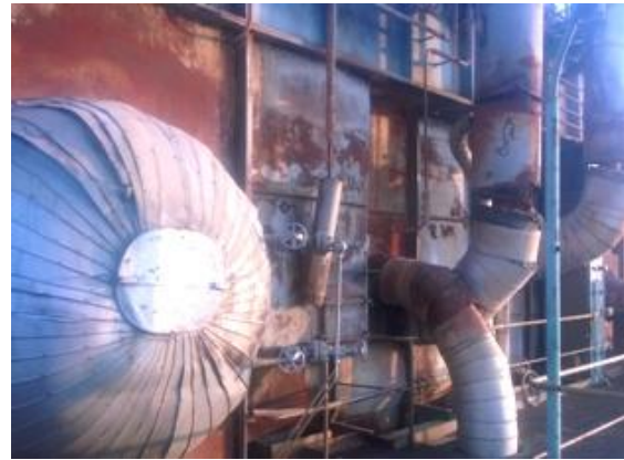
Photo 3-9 Boiler top and Drum
