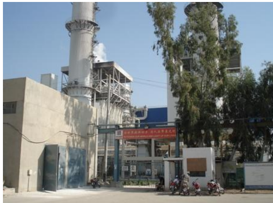
Photo 3-1 Facility of gas turbine and HRST
