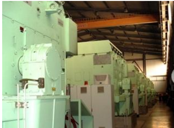
Photo 7-2 Diesel engine generator
