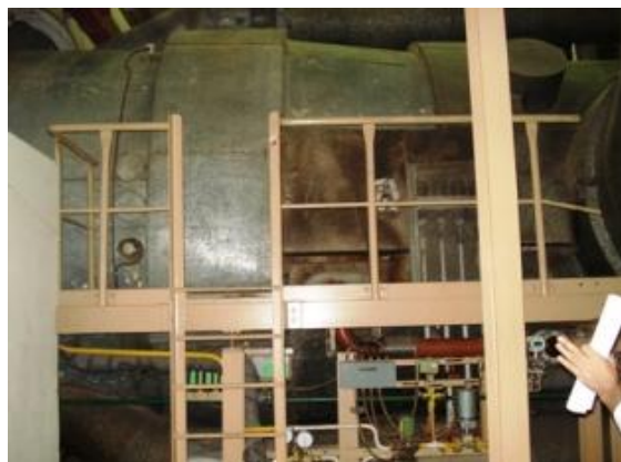
Photo 5-6 Gas turbine combustor
