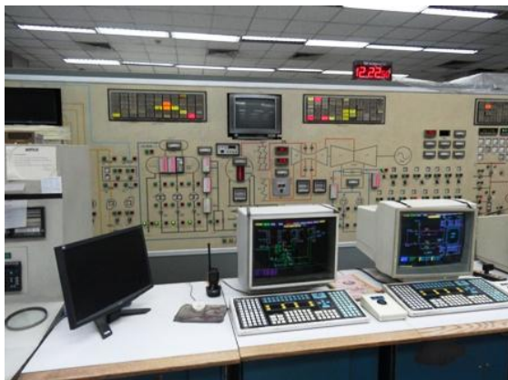
Photo 2-3 Plant console desk for unit No.4
