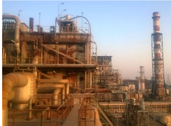
Photo 3-7 Steam boiler (left) and Stack
