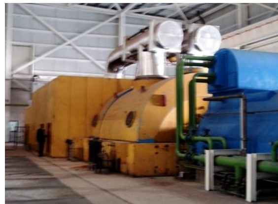
Photo 3-2 Steam turbine and generator
