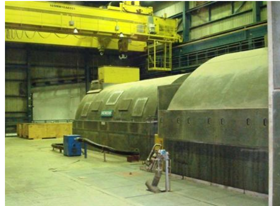
Photo 4-2 Steam turbine generator
