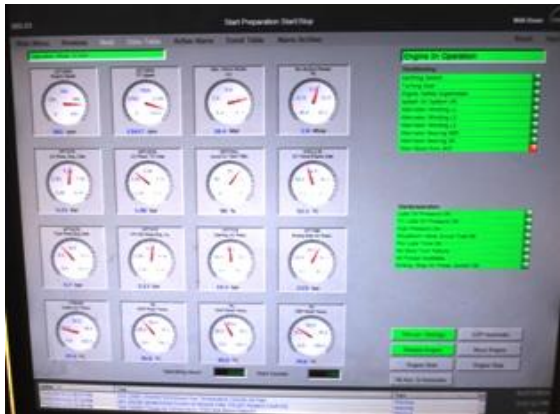
Photo 7-3 Operation monitoring system screen 1
