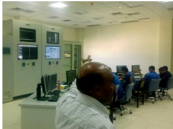
Photo 3-4 Control room for new plant
