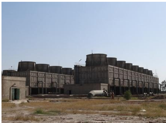
Photo 2-5 Condenser cooling tower
