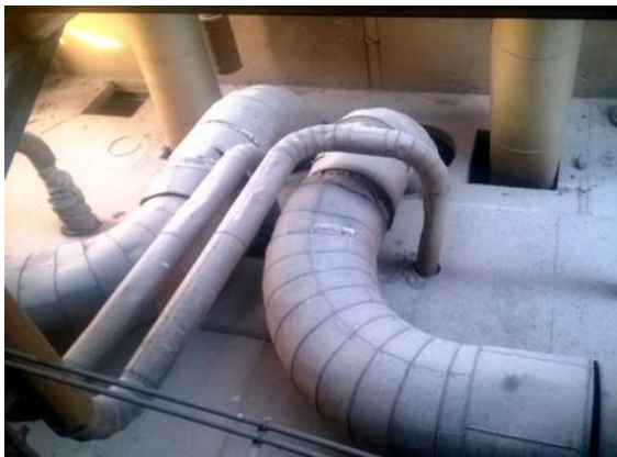
Photo 3-8 Heat insulation for steam pipe
