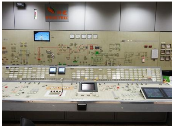
Photo 1-6 The console desk for Unit No.1
