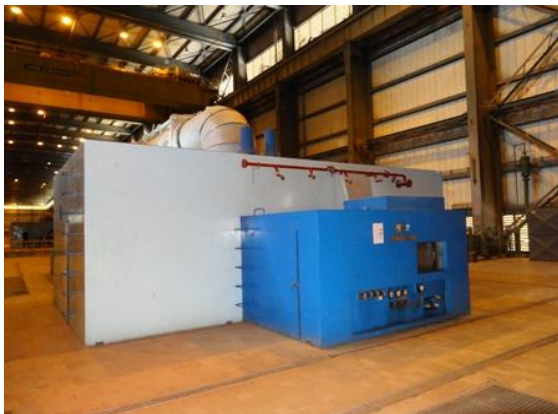
Photo 1-3 No.1 Turbine form the top side
