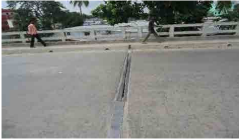
Damaged Expansion Joint (Not Damaged in Main Structures)
