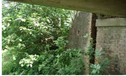
Crack at wing wall
