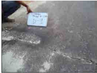
Crack in Slab
