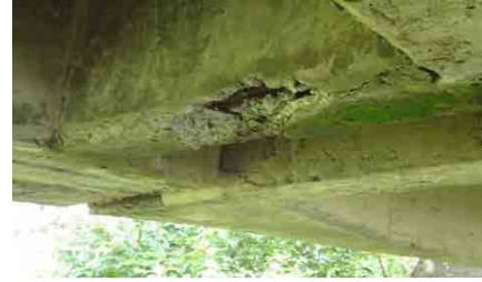
Spalling at girder
