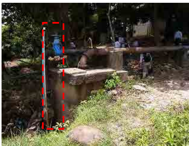
Photo 1.4.5-2 Water Gauge at Intake Station
