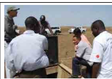
The Kassala SWC staff visited main raw water transmission line from the well field to Hawata town.
