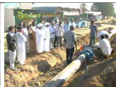
The ground-breaking ceremony of the pipe replacement. Attendant: State government, Ministry of physical planning, SWC Director General, JICA evaluation team (January 19, 2014)
