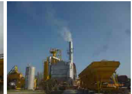
General view of dust collector (Part2), dust from the chimney
