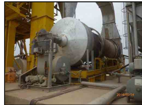
Dryer and dryer burner
