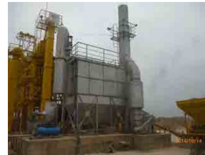
General view of dust collector (Part1)
