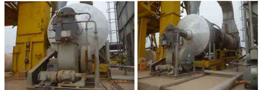
Front view of Dryer burner
