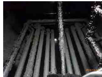
Heat piping at asphalt tank
