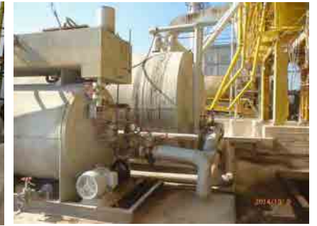
Vicinity of hot oil circulation pump
