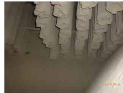
Inside bag filter (some torn filters)
