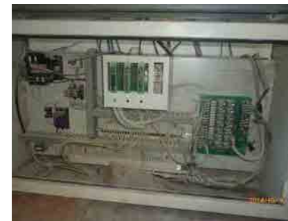
Newly replaced load cell amplifier
