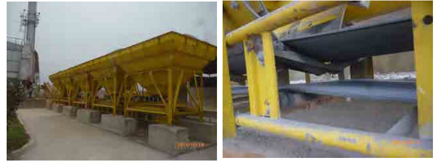
Cold bin, Belt feeder, Belt conveyor
