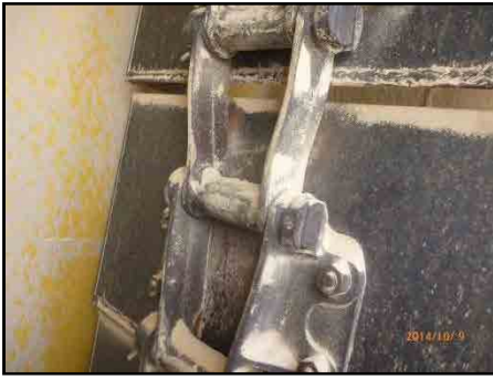
Quite few wear at the chains of hot elevator
