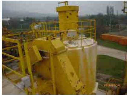
Top of filler silo, Upper part of filler elevator
