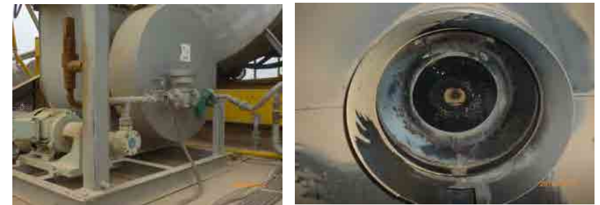
Vicinity of the pump
