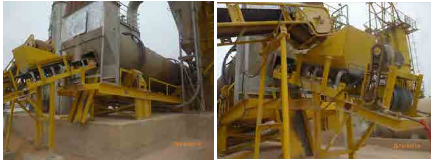
Cold aggregate conveyor, Dryer
