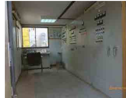
Control room inside
