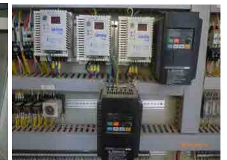
Newly replaced inverter
