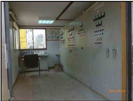
Inside the control room
