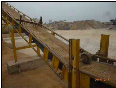
Bending spot of belt conveyor
