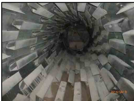
Good conditioned turbines of dryer burner
