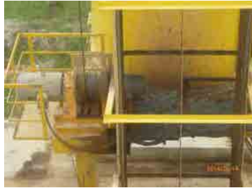
Spilled asphalt mixture is building up near the winch.
