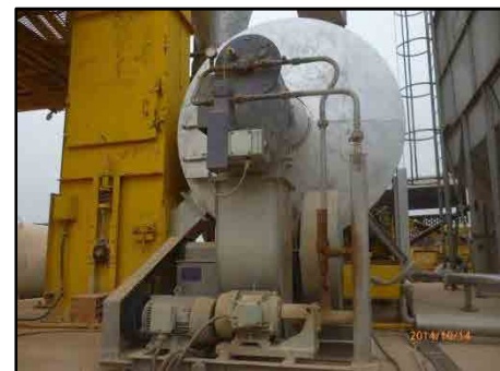
Pressure gauge at the dryer burner
