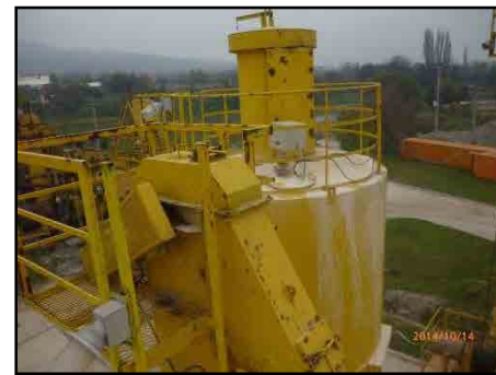
Locally installed sounding leveler at filler silo
