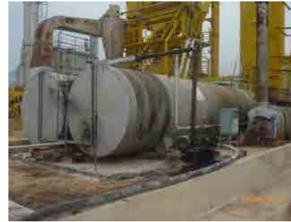
General view of asphalt supply system
