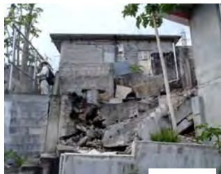
Landslide in Vall Photo
