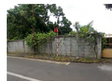
Crack on the wall (near the school)
