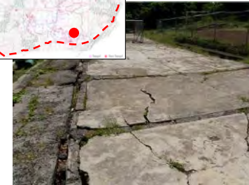
Crack (behind the school)
