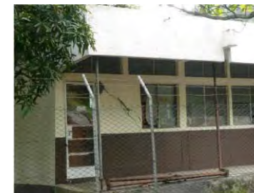
Damage of the school
