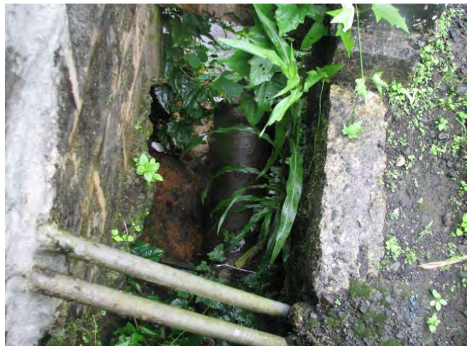
Eroded area the eroded depth is 50cm
