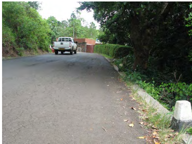
Crack on the road side
