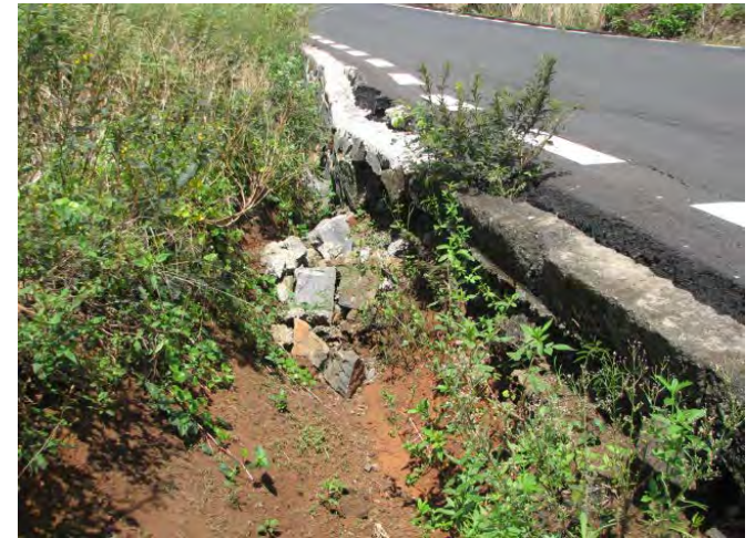
Erosion of foundation
