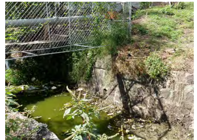
Cracks at bank protection
