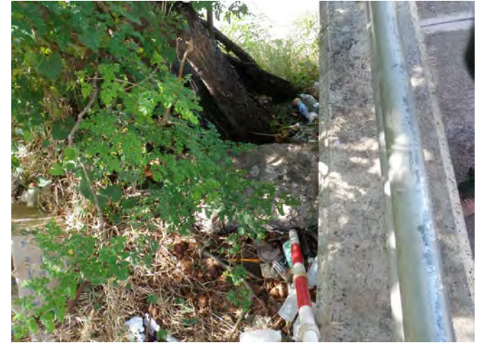
Crack of concrete
