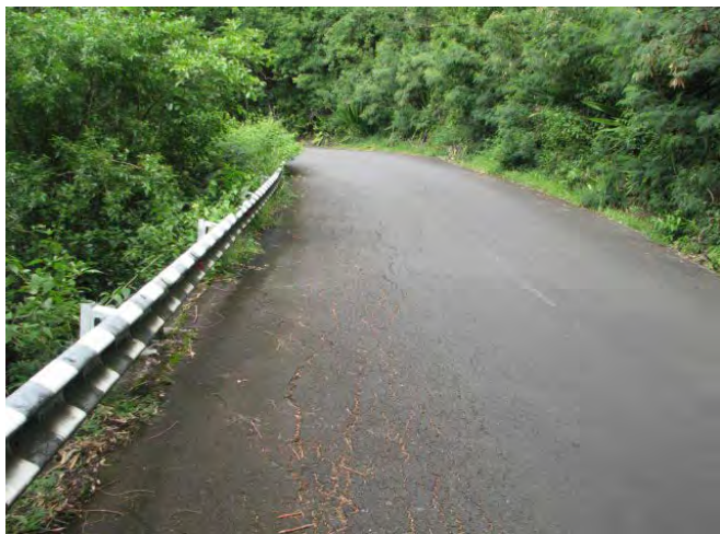
Cracks and subsidence along A-A' line
