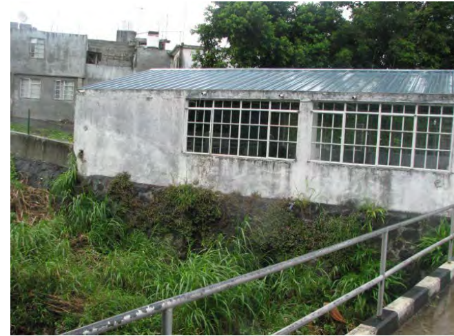
High water overflow at the bottom of the building
