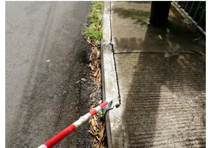
New crack along the road
