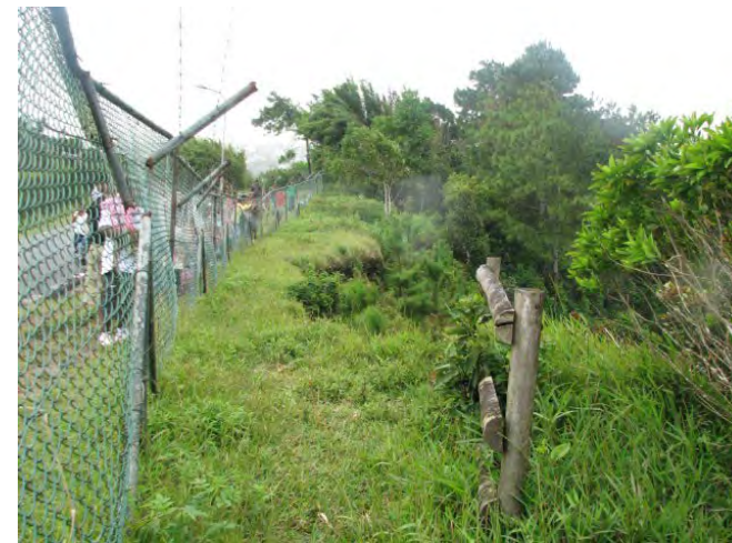
The top of the slope failure
