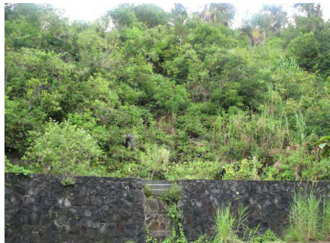
Trace of past slope failure
