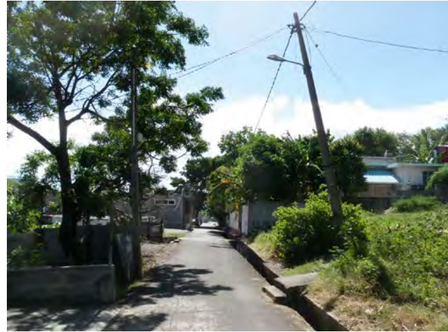
Incline of a telephone pole
