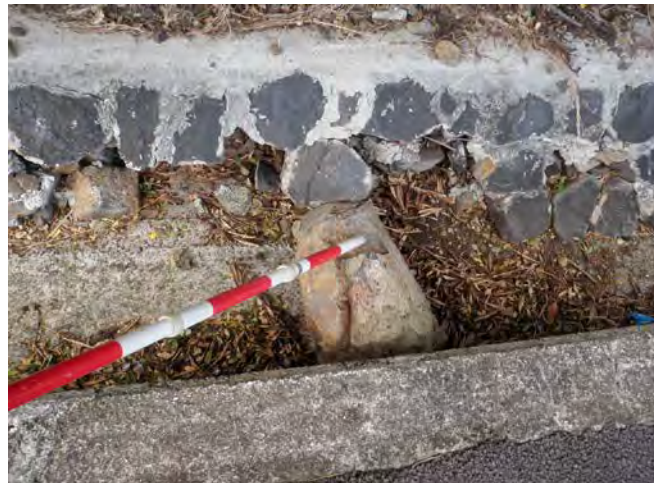
Rockfall from the mountain
