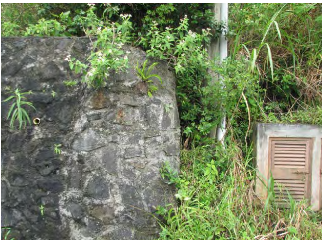
Cracks on retaining wall
