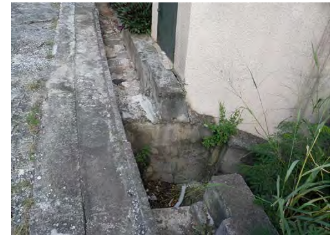
Damage on house
