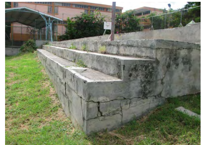
Horizontal cracks of the concrete step
