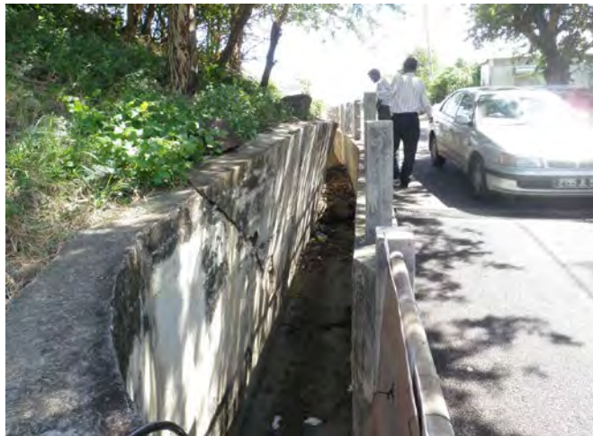
Inclined the retaining wall
