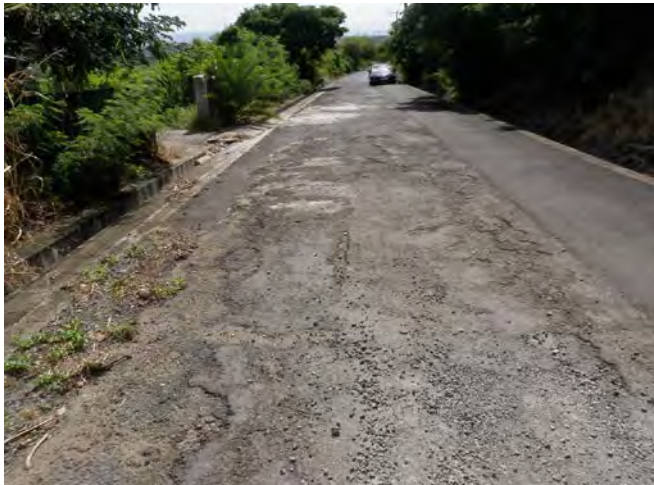
Cracks on the road
