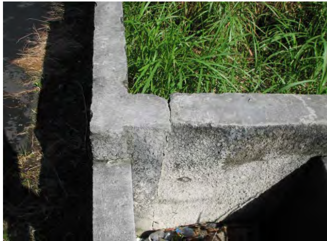
Crack of concrete wall
