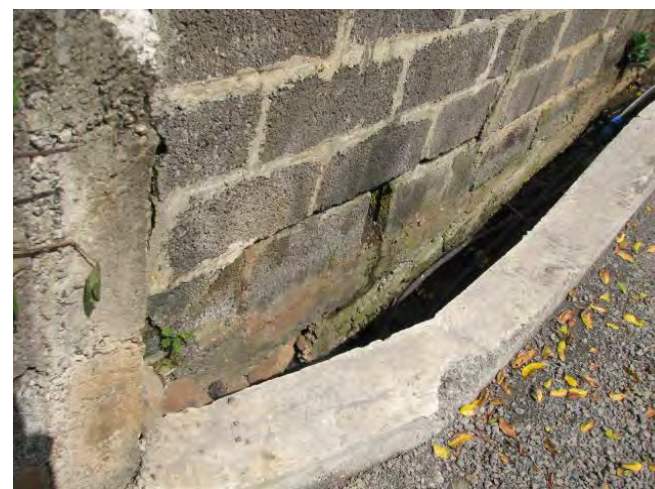
Damage of the drainage of the roadside
