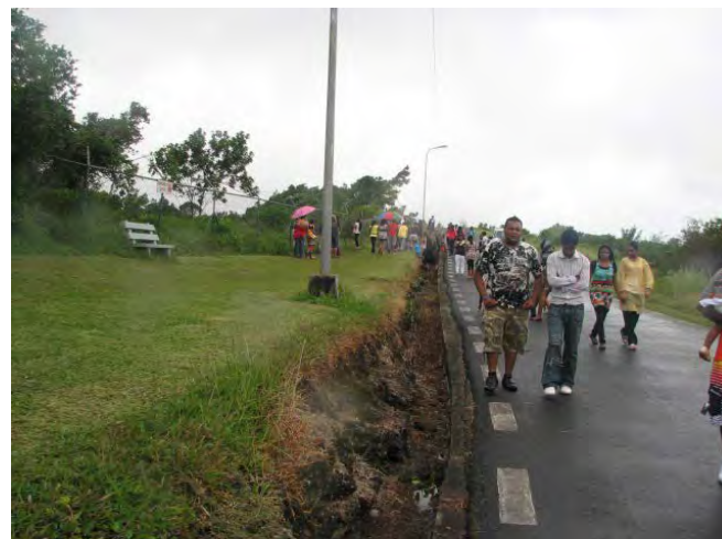
The back of the slope failure
