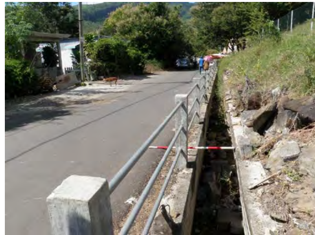
Inclined the retaining wall
