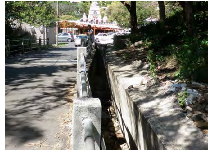
Inclined the retaining wall
