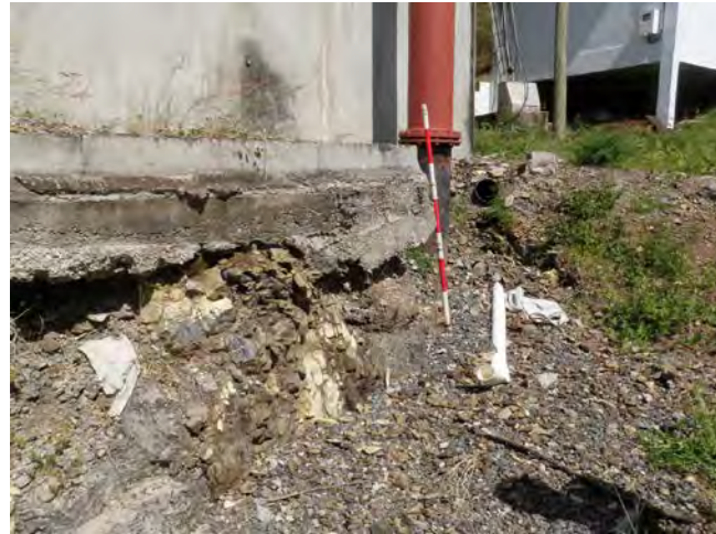
Erosion of the tank foundation
