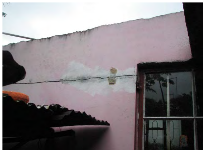
Heavy damages at houses
