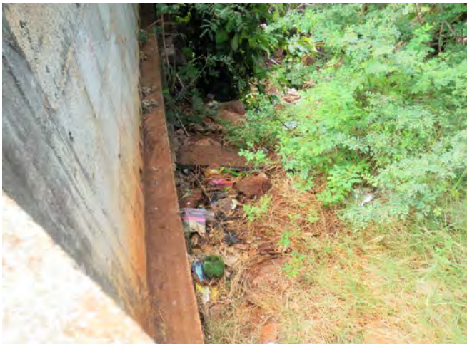
Erosion around structure
