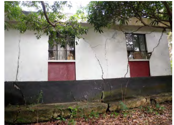
Heavy damage at houses
