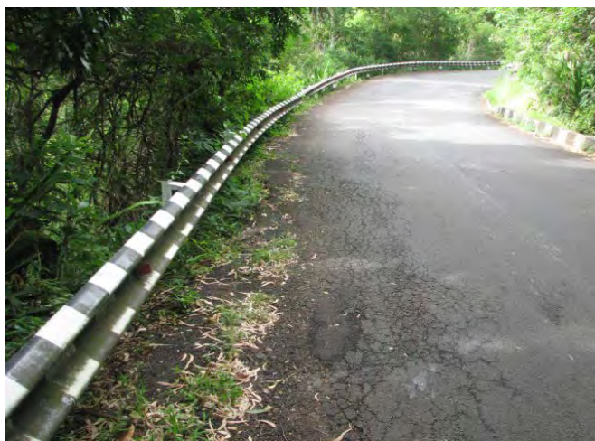
Cracks and subsidence on lower part
