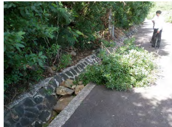
Rockfall from the mountain
