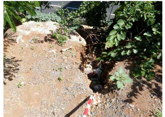
Top of trace of erosion
