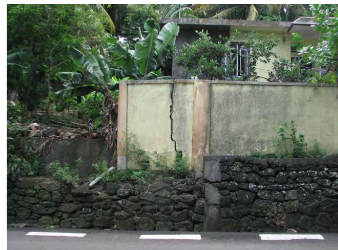
Heavy damages at houses
