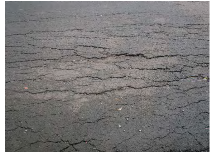
The crack occurred in the road shoulder (by damage of differential settlement)
