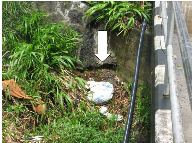
Erosion at the bottom of the building
