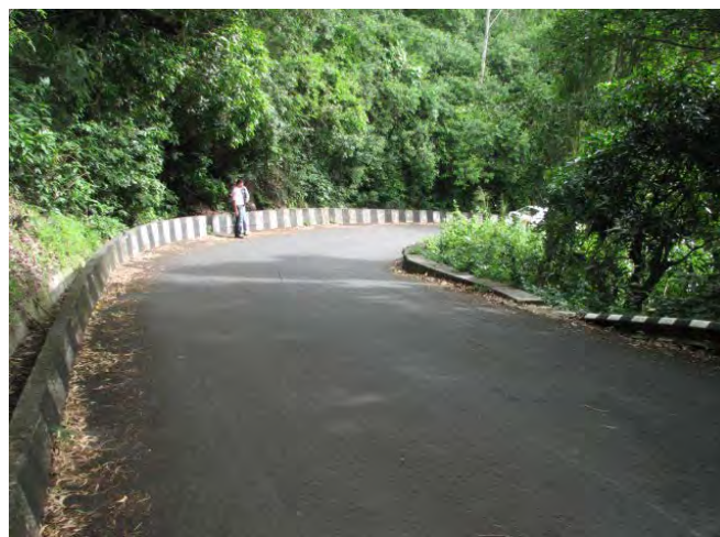
Cracks and subsidence along B-B' line
