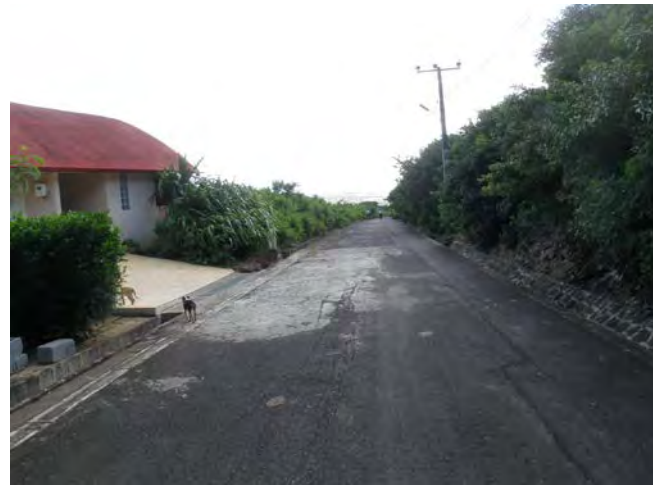
Cracks on the road
