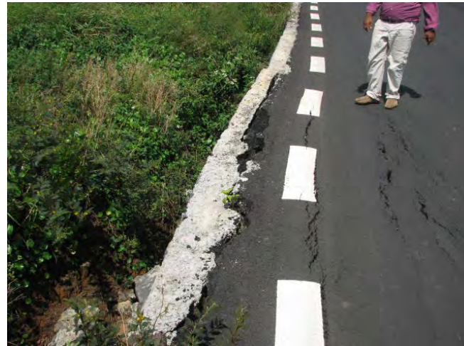
Deformation by erosion of foundation
