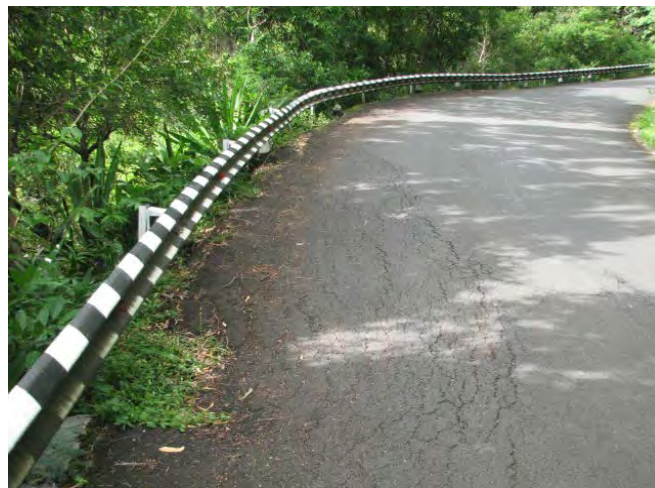
Cracks and subsidence on upper part
