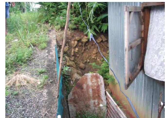
Small collapse next to the house
