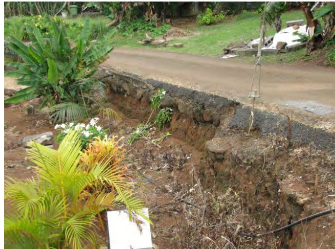
Damage in retaining wall by erosion
