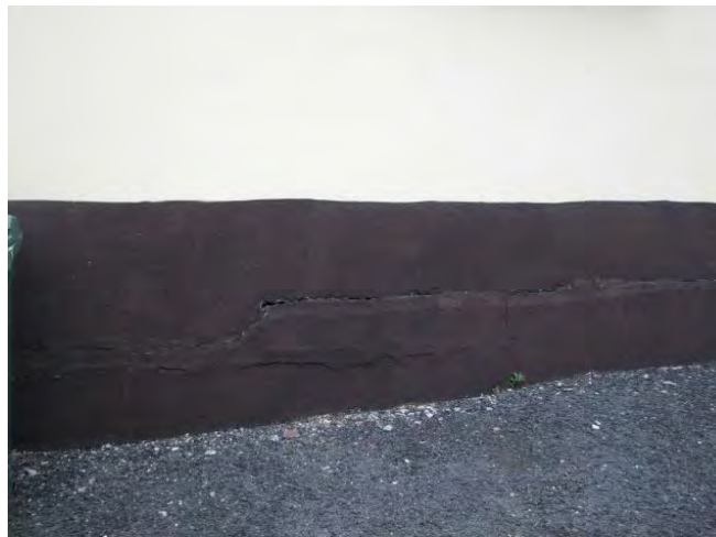
Cracks on wall
