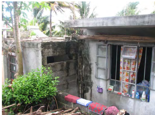
Heavy damages at houses
