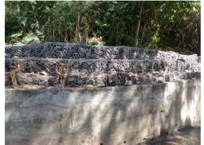
Some gabions have been damaged a little.
