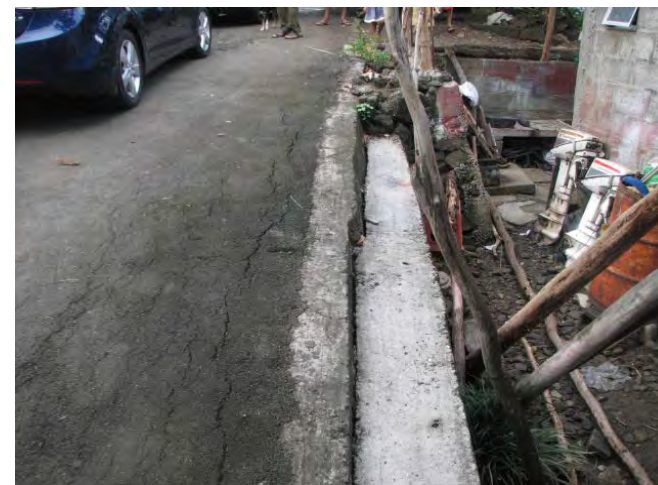
Head cracks of the lower landslide
