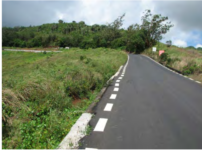
Full view of the damaged road
