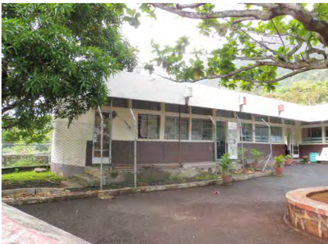
Heavy damage at school
