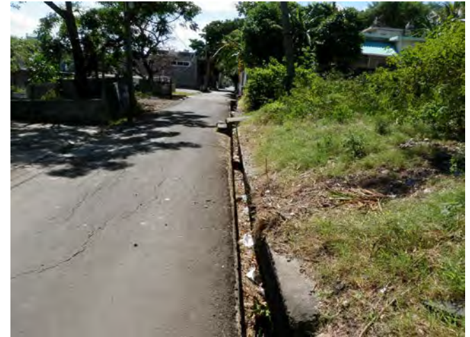
Retaining wall incline (Pushing of back out)
