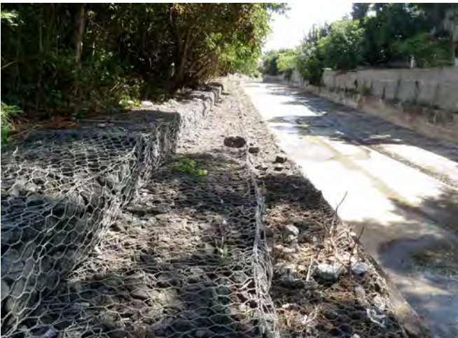
Some gabions have been damaged a little.
