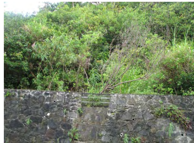
Trace of past slope failure
