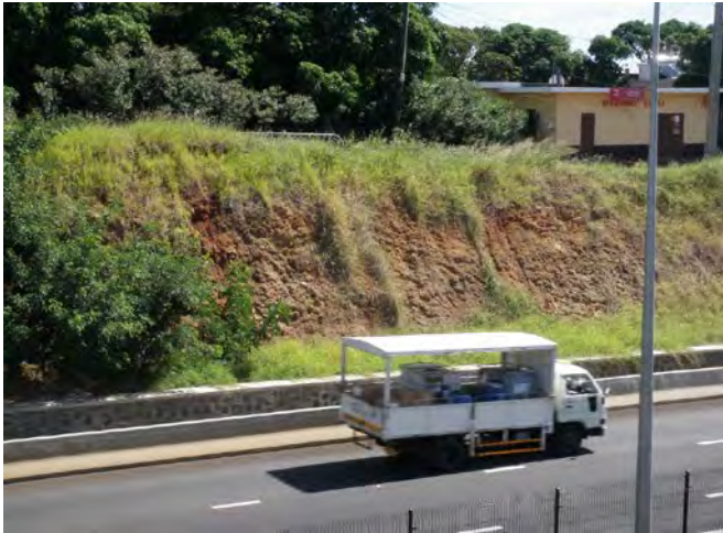
Full view of the slope failure
