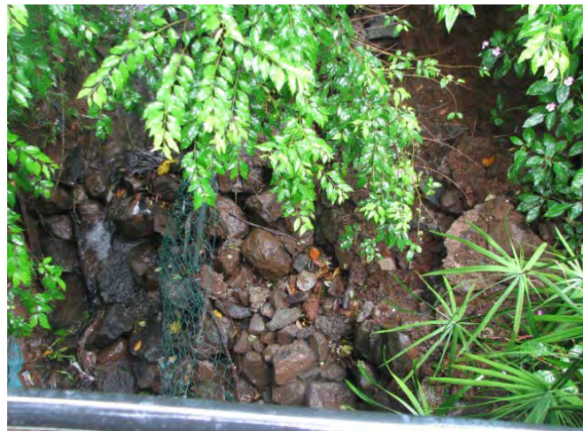
Close view of collapsed rocks
