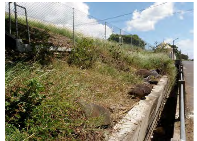
Inclined the retaining wall
