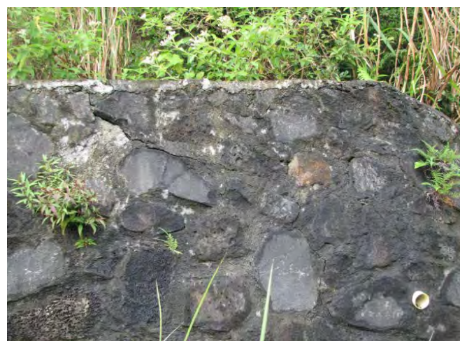
Cracks on retaining wall
