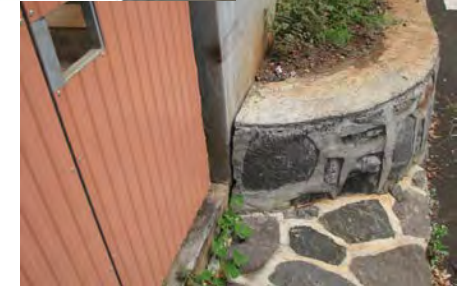
Cracks around the house
