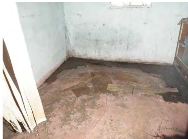
Spring water in corner of basement
