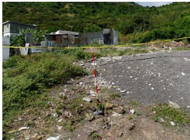
New cracks observed behind the house
