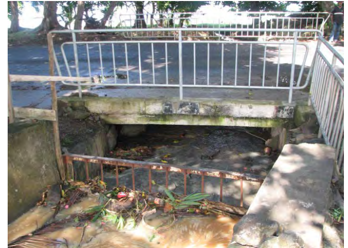
Inlet of the box culvert Small debris and garbage are stacked
