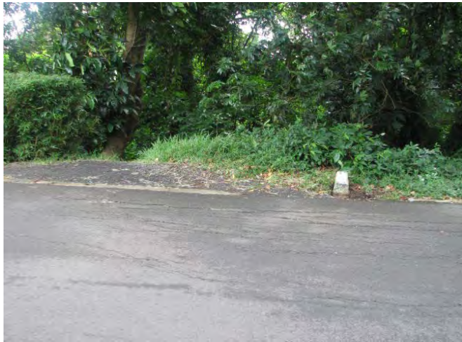
Crack on the road side
