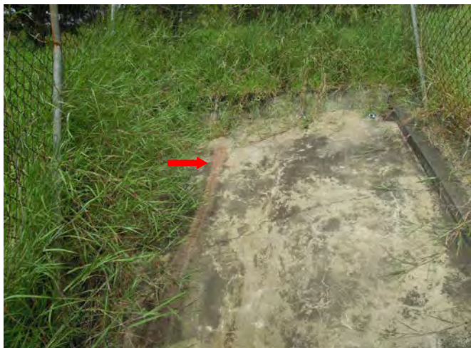
Horizontal drilling. The brown trace of water-flow was identified (red arrow)
