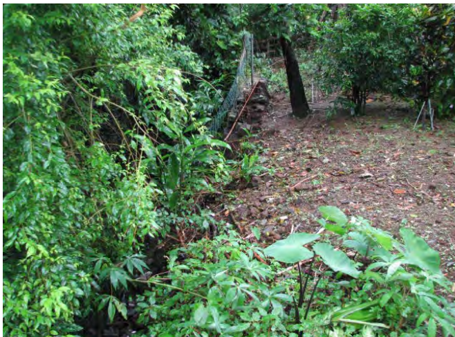
Broken wall on house side
