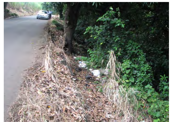
Rocks and gravel by slope failure
