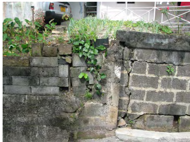
The damage of the concrete block wall
