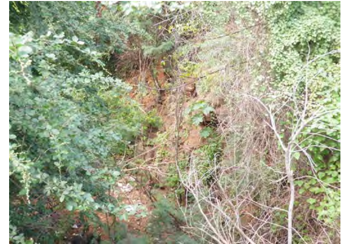
Bank erosion around bridge abutment
