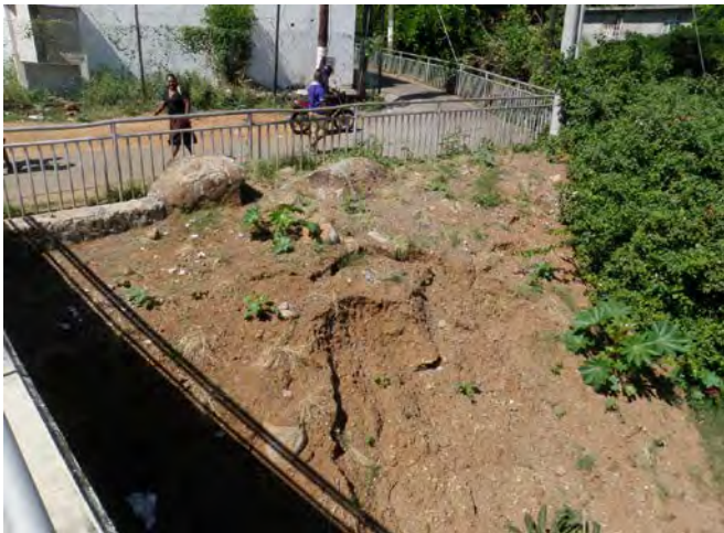
Full view of the slope failure( New failure)
