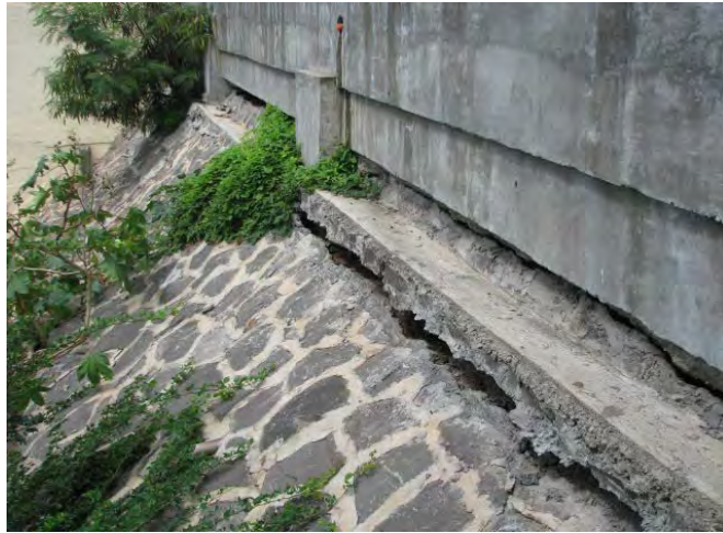
Cracks on stone block
