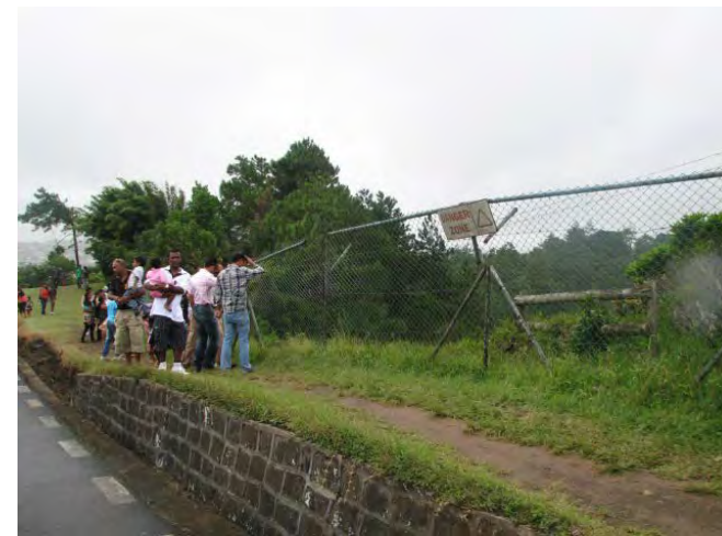
The fence in the back of the slope failure It is damaged by the slope failure
