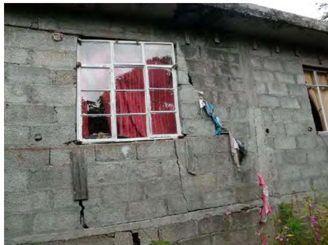
Heavy damage at houses
