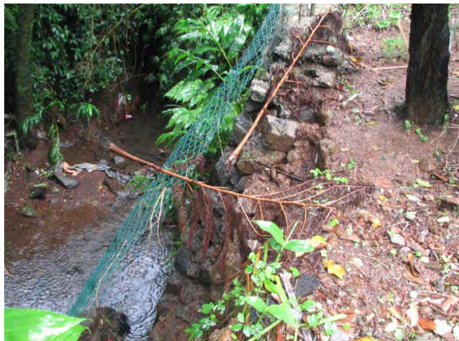
Close view of broken wall
