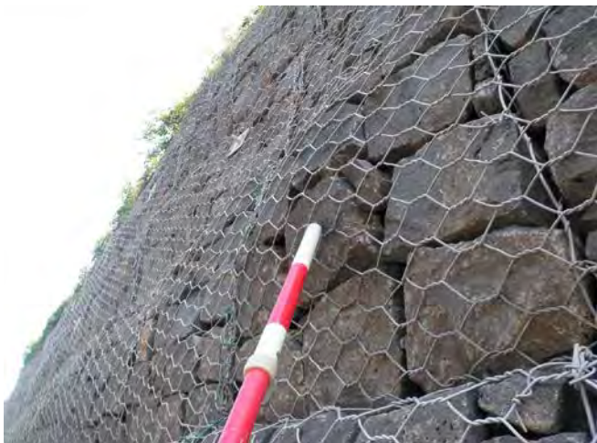
Pushing out is confirmed a little.
