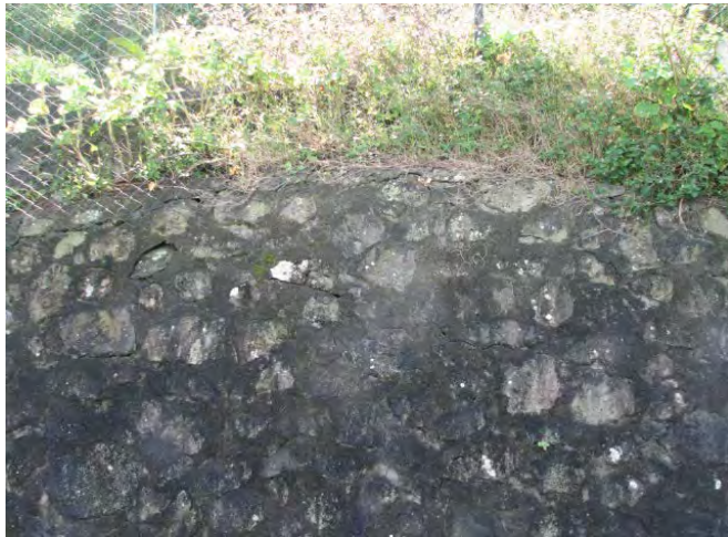
Crack of retaining wall
