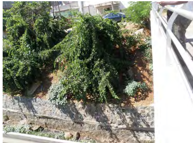
Falling rocks from the slope
