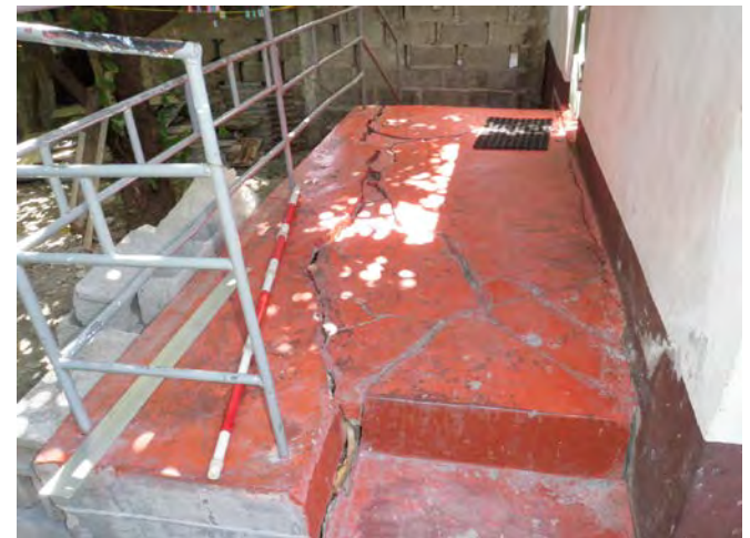
Open cracks of veranda
