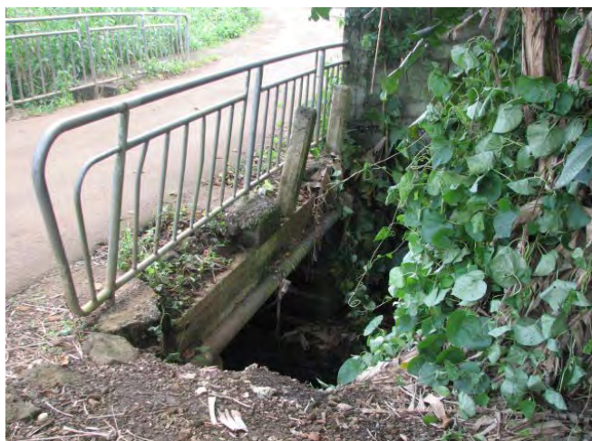
Eroded area at the upper side
