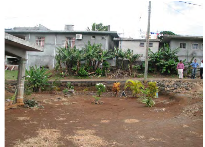
Damage in retaining wall by erosion
