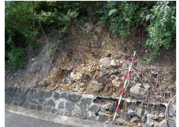
Slope failure along the road
