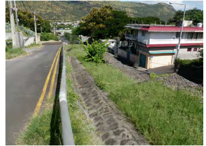
The upper part and the rear of the Gabion wall (East side)
