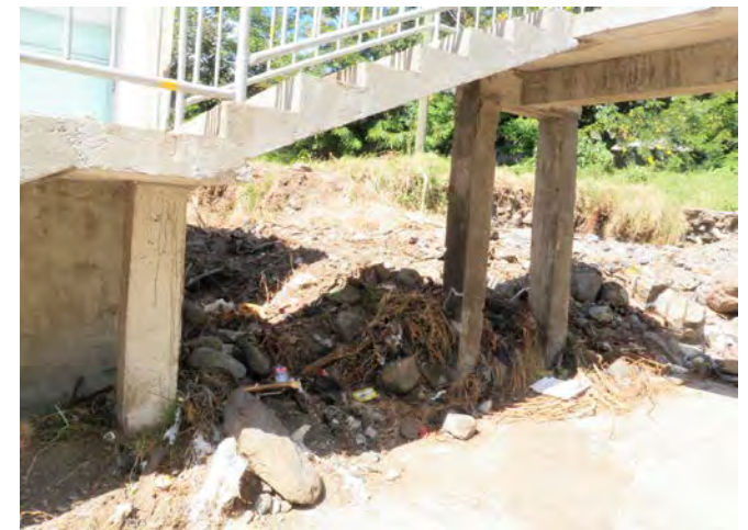
Deposited sand by debris flow
