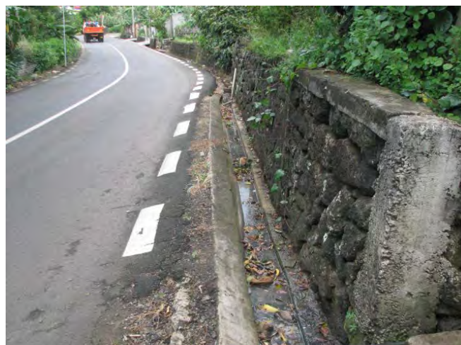
Deformed road side at the bottom of the lower landslide
